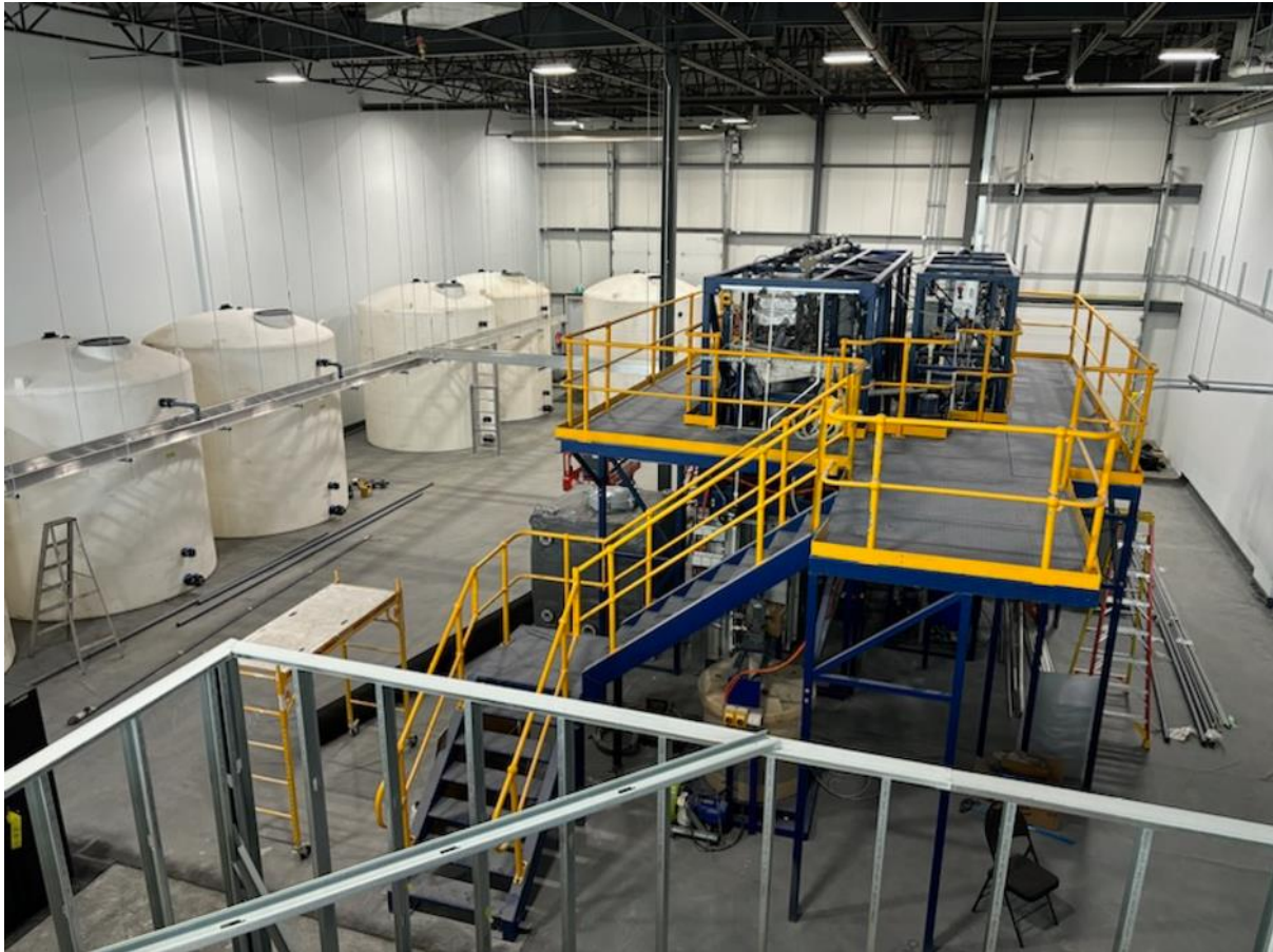
Figure 1: LithiumBank's 10,000 L/d pilot plant in the final stages of construction. Photo dated March 28, 2024
