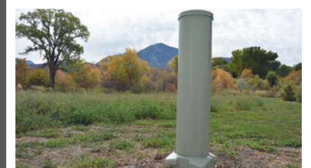
A fiber termination pedestal—big-city technology, country views.
