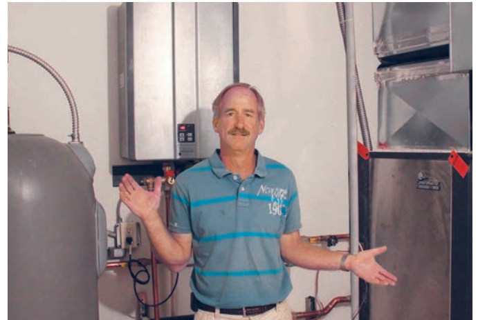
Above: Kelly Crippin stands between his new Marathon water heater and his new GeoExchange heating and cooling system.
