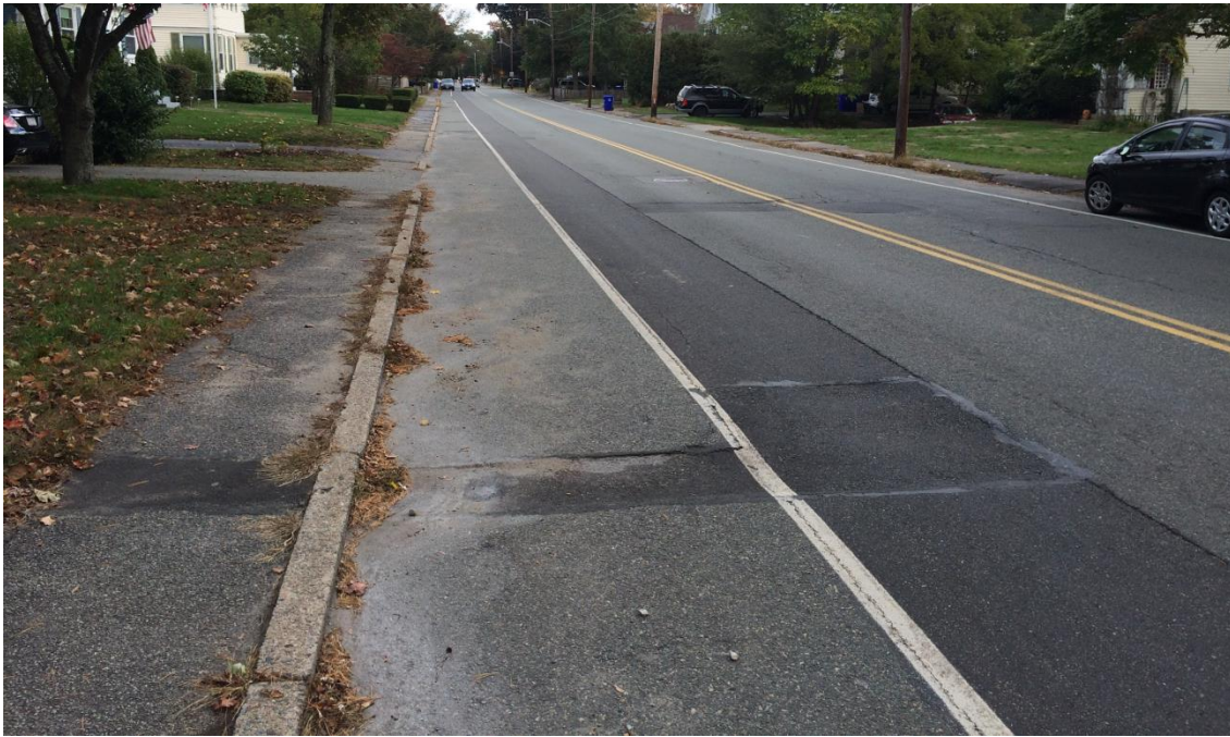
Figure 1. Pavement patch over a stretch of replaced gas main (darker pavement running length of street) and replaced service (darker pavement extending into sidewalk). At least two new seams for water, ice, and dirt to penetrate have been created running almost the entire length of the road.
