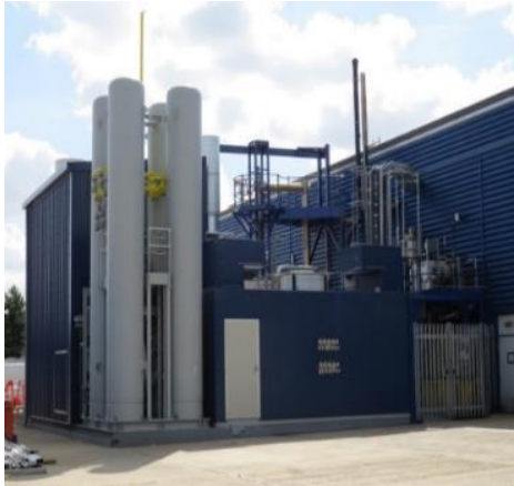
The "Gogreengas" Pilot Plant, Swindon, UK
