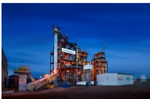
Enerkem Plant in Edmonton, Canada
