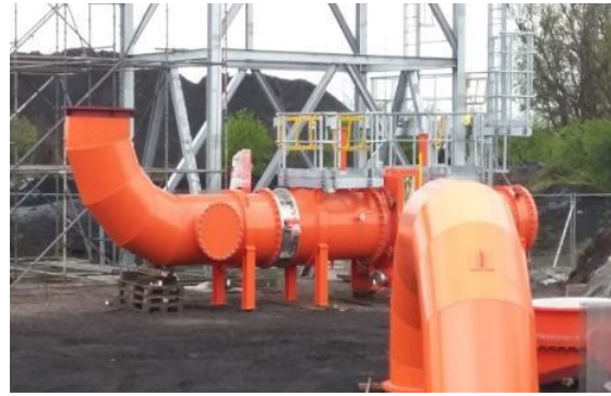
LanzaTech's Plant in Ghent, Belgium
