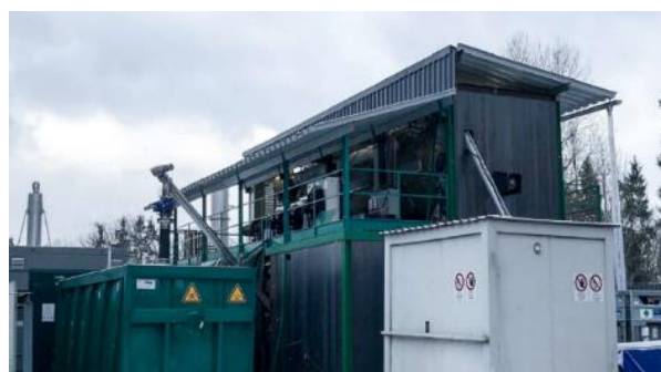
TCR300 plant, Sulzbach-Rosenberg, Bavaria, Germany
