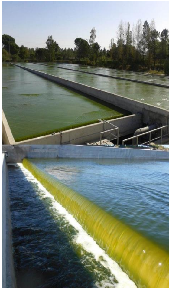
BIOFAT Pataias Pilot Plant Cascade Raceway – 2 x 1,500m 2 – Designed and built by A4F. (BIOFAT FP7 project)
