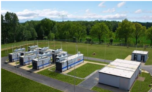
Falkenhagen Hydrogen production and grid injection, Germany
