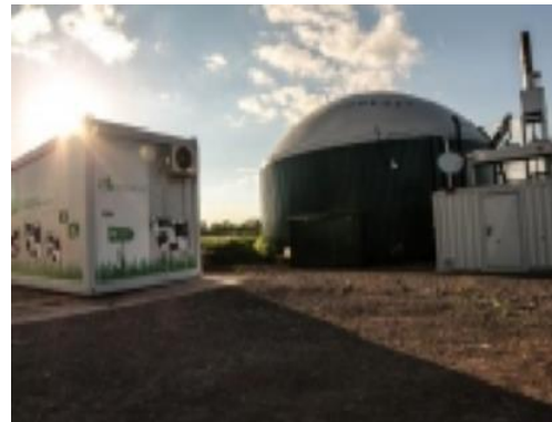
Biomethane plant of Biogest Biogas/Greener for Life Ltd in Somerset, the UK
