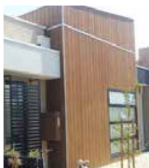
4 MONTHS: The board shows signs of lightening.
