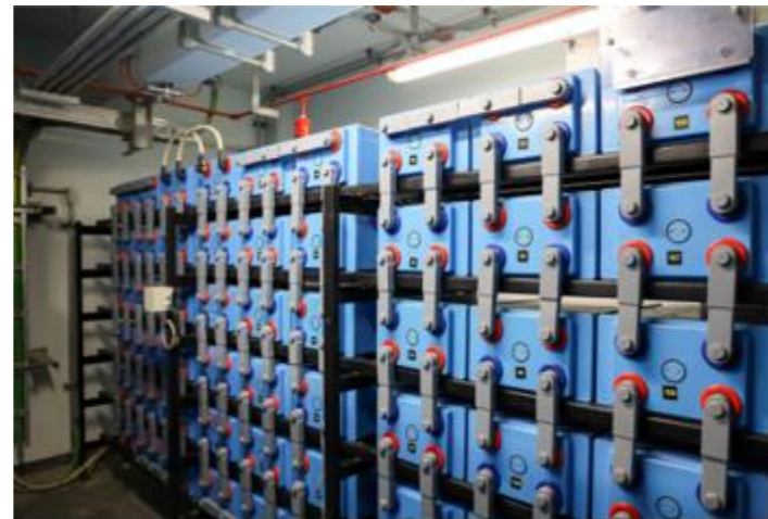
Renewable Energy Storage
