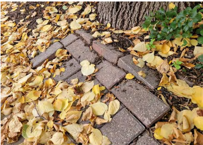
Unlevel paver surface adjacent to tree roots
