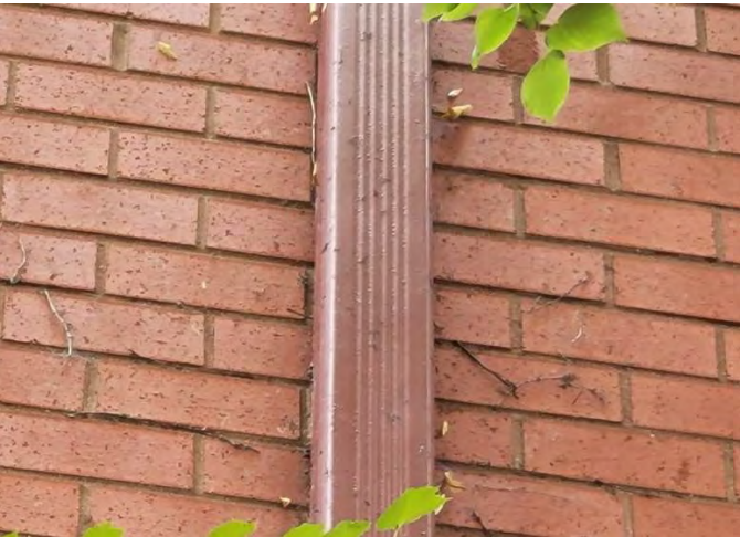
Aluminum downspout leading to grade
