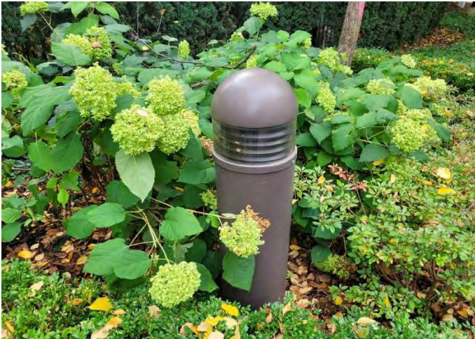
Overview of bollard light fixture
