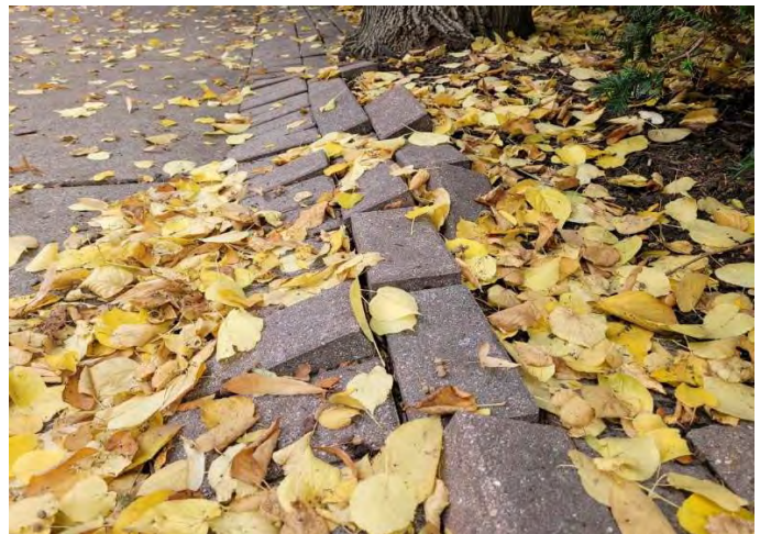
Unlevel pavers adjacent to public walkway
