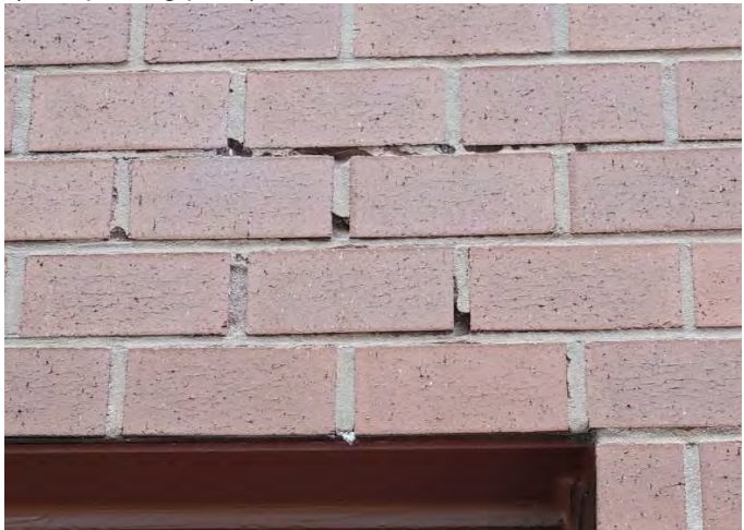
Deteriorated mortar joints in need of repointing
