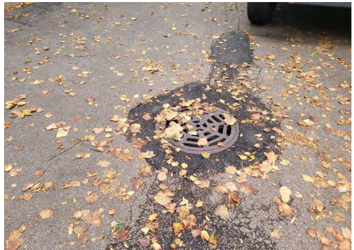
Catch basin with patched asphalt surround
