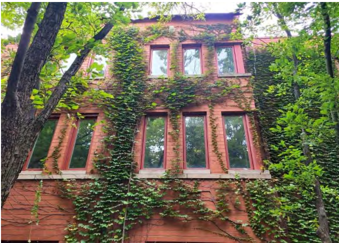
Ivy coverage at masonry façade
