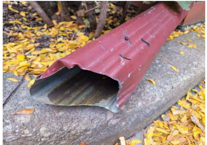
Crushed downspout extension
