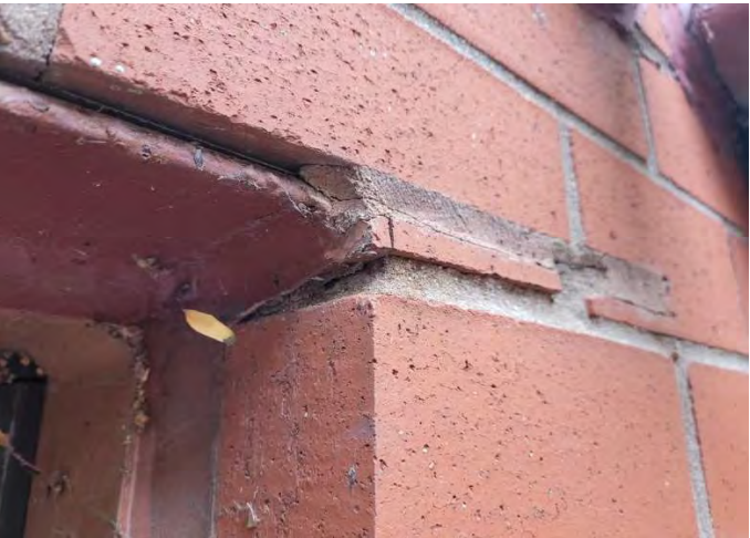
Cracked mortar at lintel bearing location
