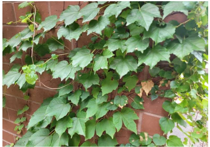
Ivy at masonry façade
