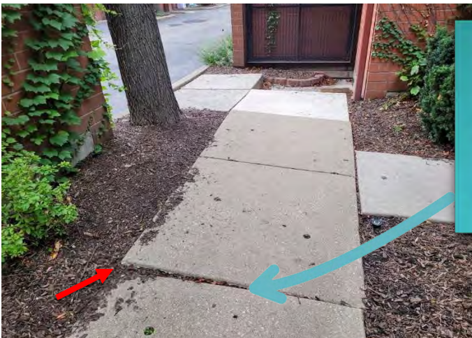
Varying ages of concrete panels; Significant trip hazard
