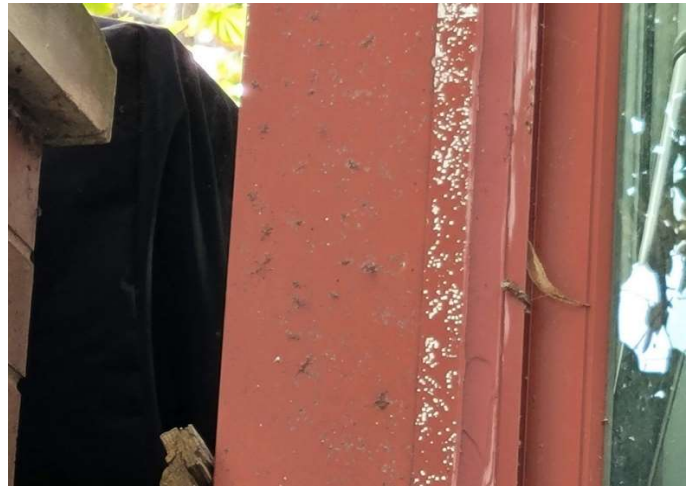
Finish deterioration at metal window corner trim
