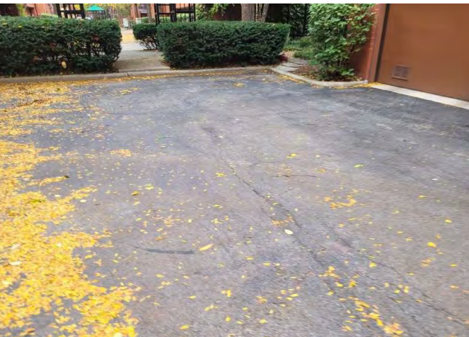
Cracking at asphalt pavement
