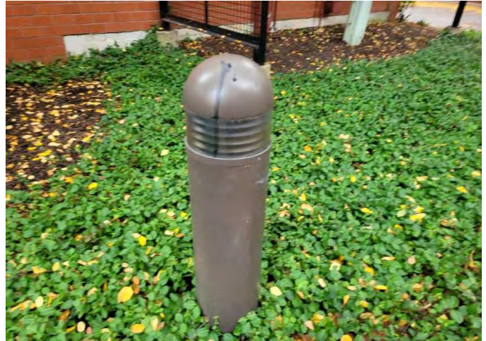
Bollard light along common walkway
