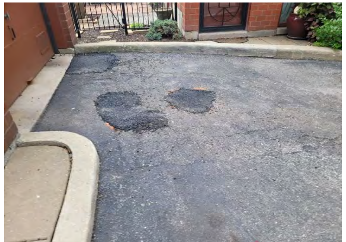
Patches, cracks, and deterioration at pavement
