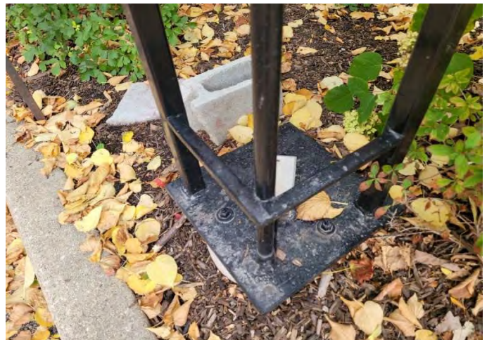
Steel lighting frame
