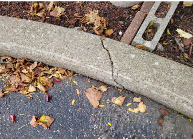
Cracked concrete curb
