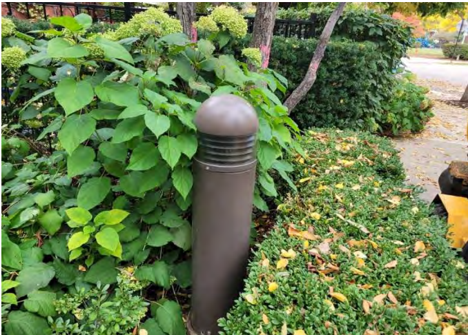
Bollard light along common walkway
