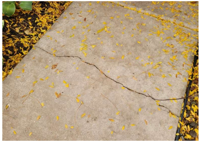
Cracked sidewalk panel
