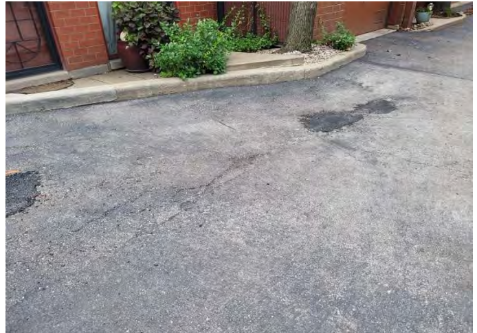
Patches, cracks, and deterioration at pavement
