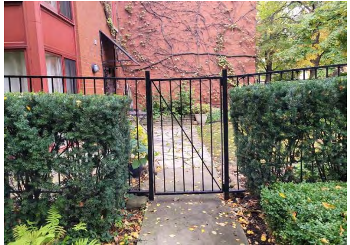
Heaved and unlevel fencing and gate
