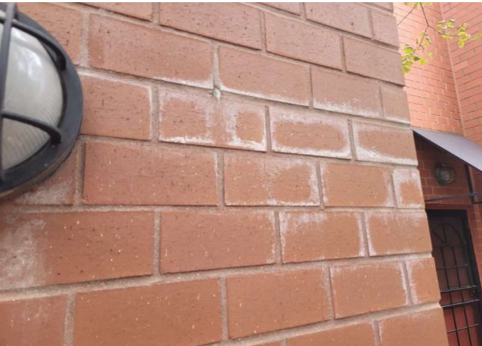
Efflorescence - sign of present or past water infiltration
