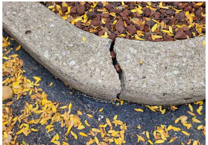
Cracked concrete curb
