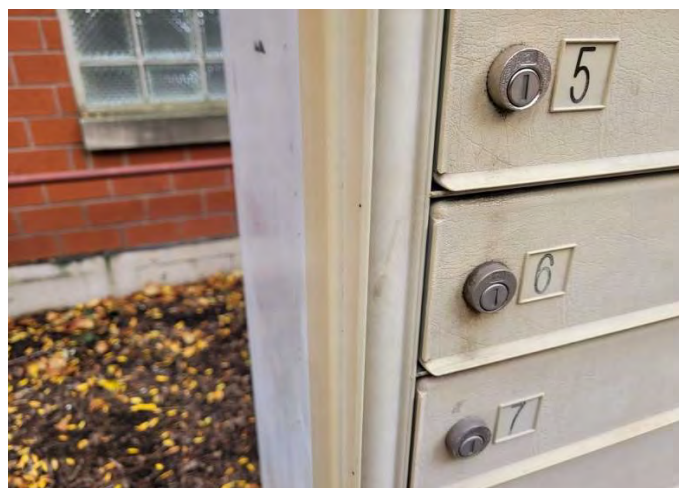
Finish deterioration at mailbox
