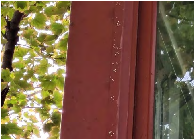
Finish deterioration at metal window corner trim
