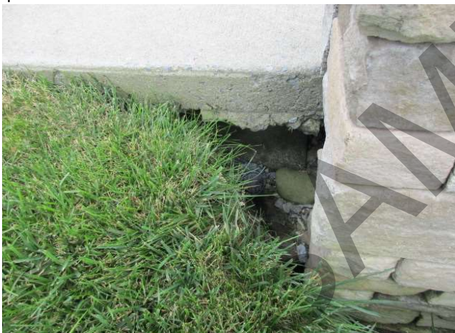
Erosion under sidewalk at BLS clubhouse north pool area entrance
