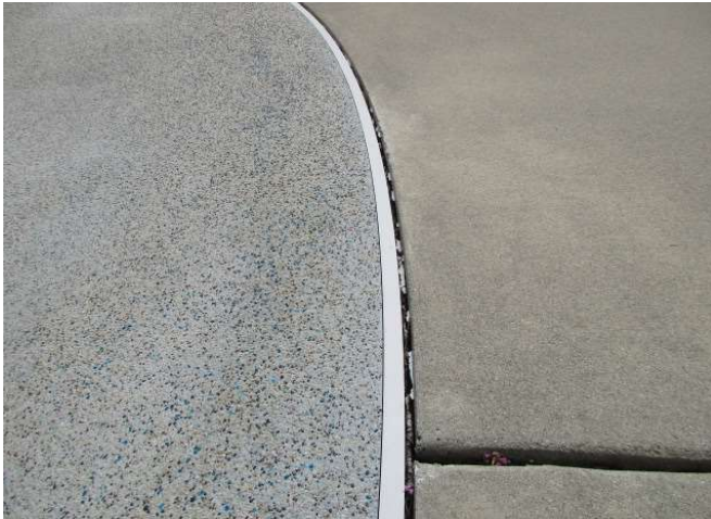
Gap between zero-depth entry and deck at BLS clubhouse pool
