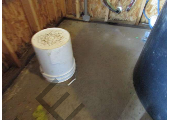
Standing water at BLS clubhouse irrigation well house
