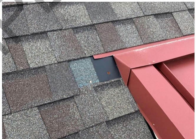
Missing shingle - photo provided by client
