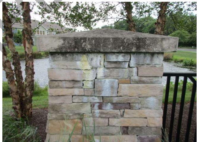
Efflorescence at entrance monument
