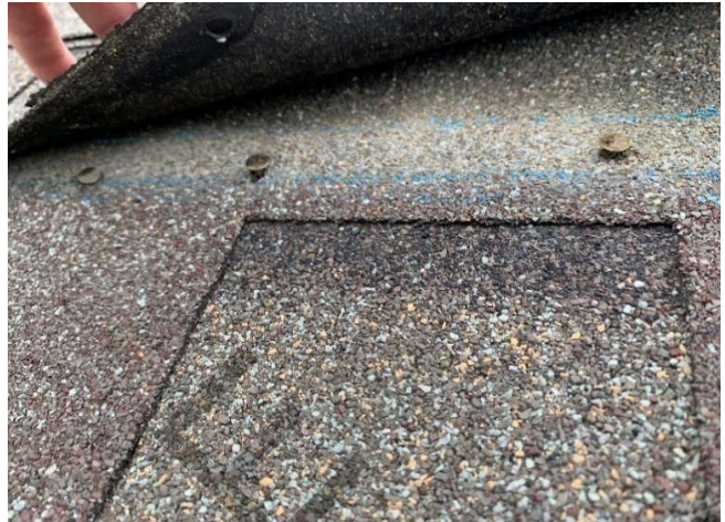
Nail pops - photo provided by client
