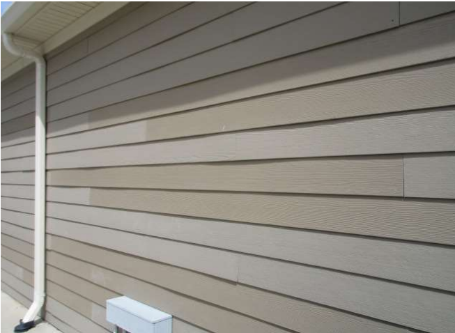
Non-matching siding at BLS clubhouse south elevation
