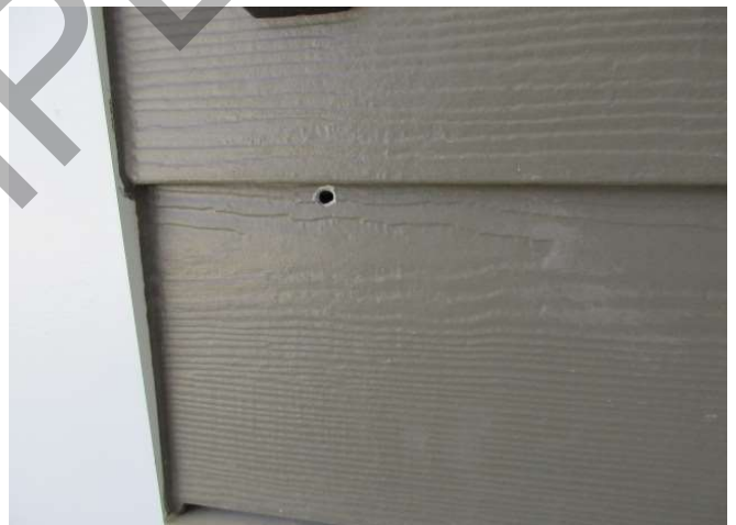
Hole in siding at BLN clubhouse near north door
