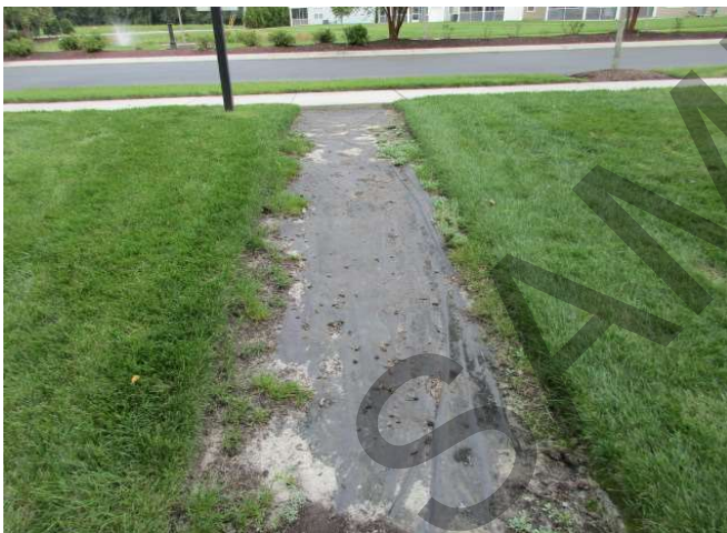
Missing walking surface
