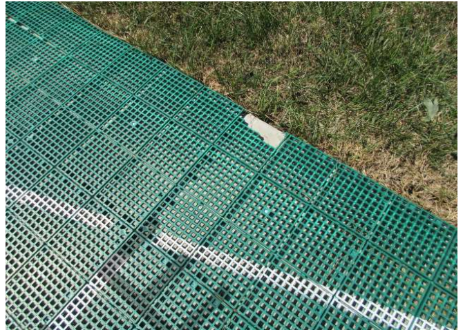
Damaged poly surface
