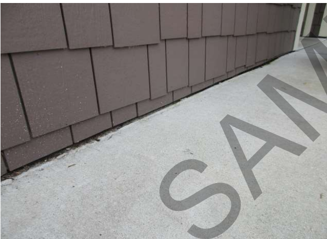
Insufficient spacing between concrete and siding
