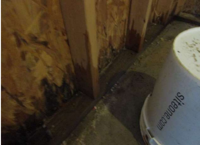
Water damage at BLS clubhouse irrigation well house
