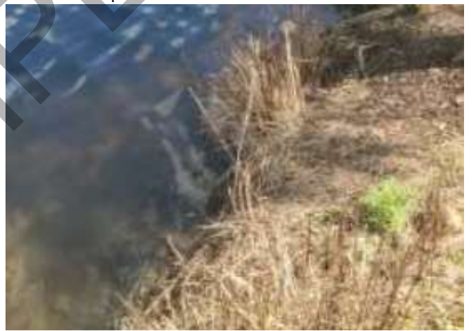
Erosion at Pond #4 behind lots #96-99 - photo from Envirotech report
