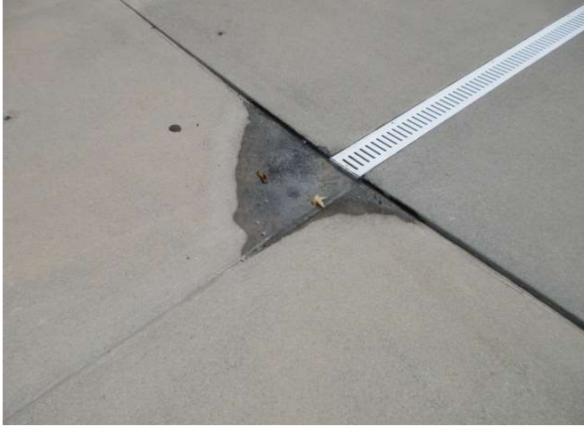
Concrete settlement at BLS pool deck
