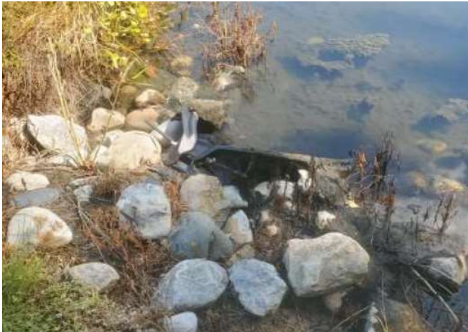
Lack of geotextile fabric at Pond #2 - photo from Envirotech report
