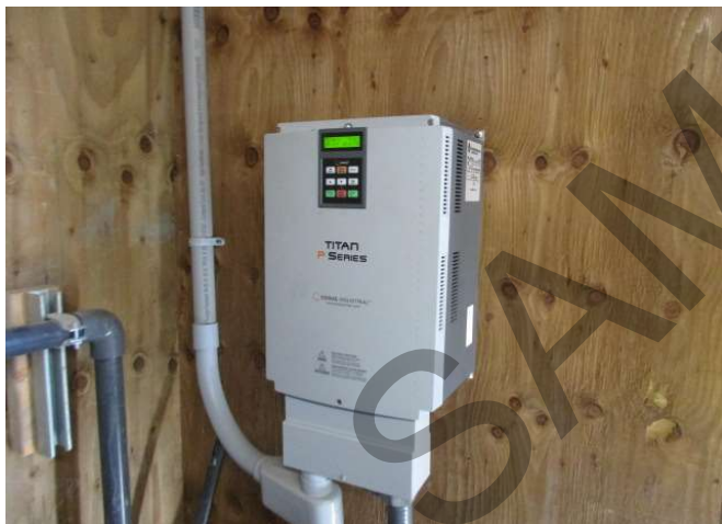
Existing BLN pump variable frequency drive
