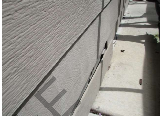
Loose siding at south elevation
