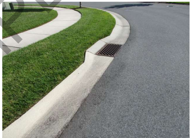
Pavement lower than catch basin entrance
