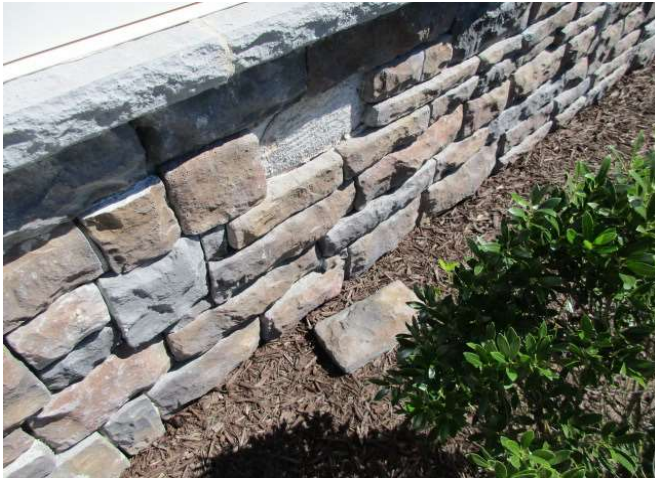
Loose stone at BLN clubhouse
