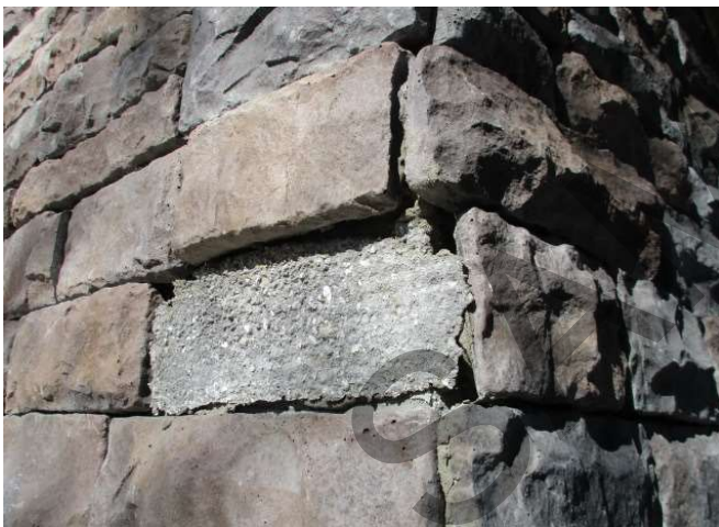
Missing stone at BLN mailbox kiosk wall
