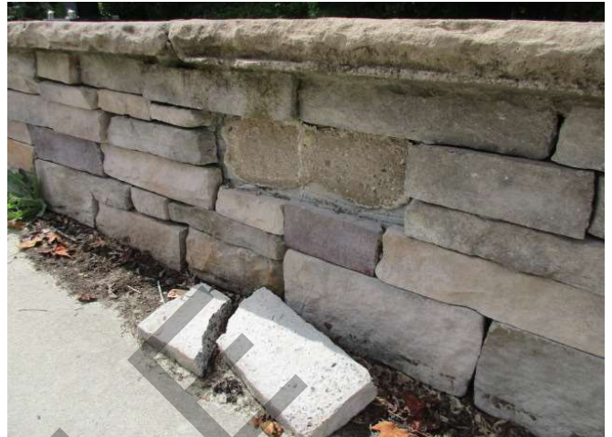
Damaged stone at BLS clubhouse knee wall
