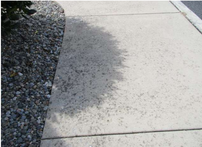
Spalled concrete sidewalk south mailbox kiosk
