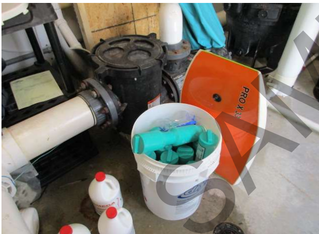
Water on floor at BLS clubhouse pool mechanical equipment room
