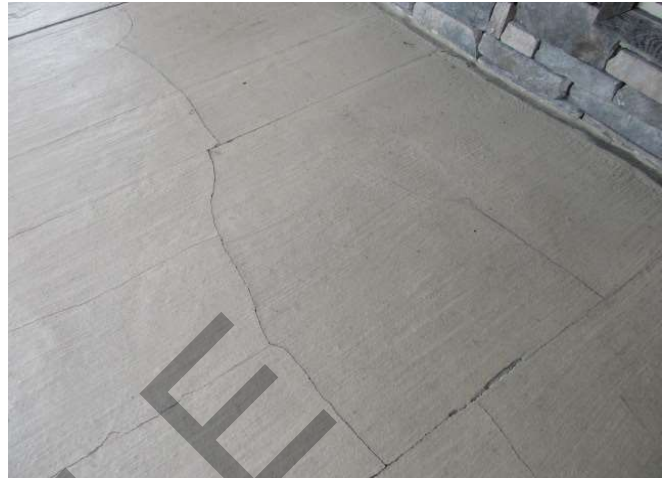
Cracked coating at south mailbox kiosk
