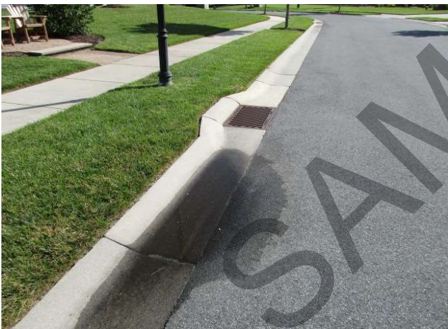
Standing water adjacent to catch basin
