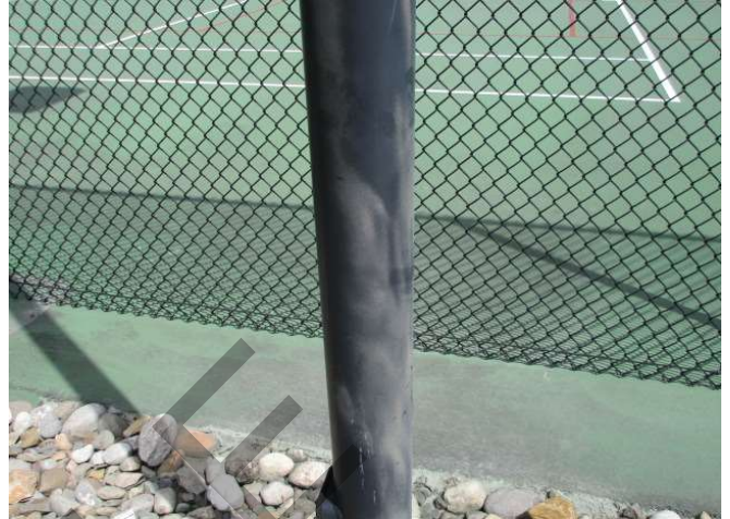
Faded finish at pole
