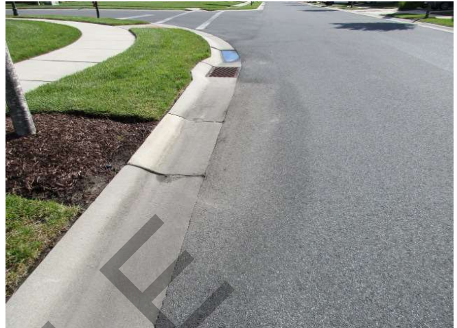
Evidence of past standing water
