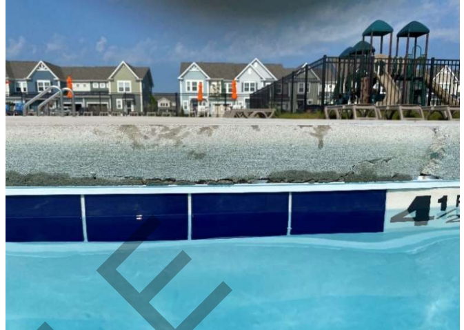
Coping deterioration at BLN - photo provided by client
