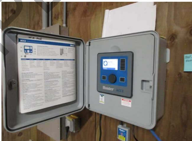
Existing BLN irrigation controller
