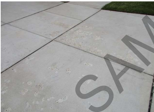
Spalled concrete driveway apron at 18201 Delafort Lane
