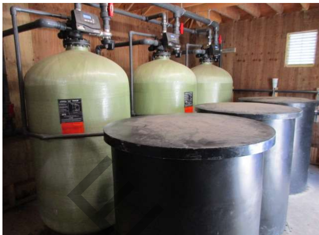
Existing BLN water treatment
