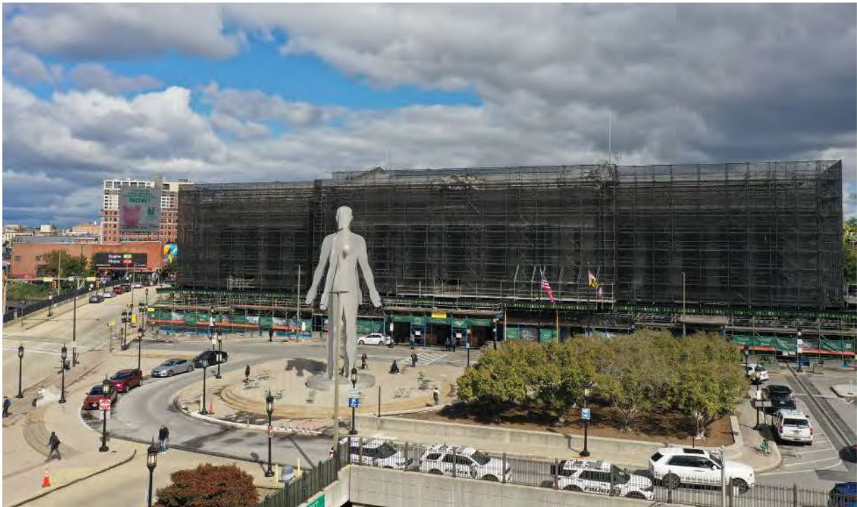
Historic Penn Station is undergoing a major transformation, including a full exterior restoration. Learn more at baltimorepennstation.com
