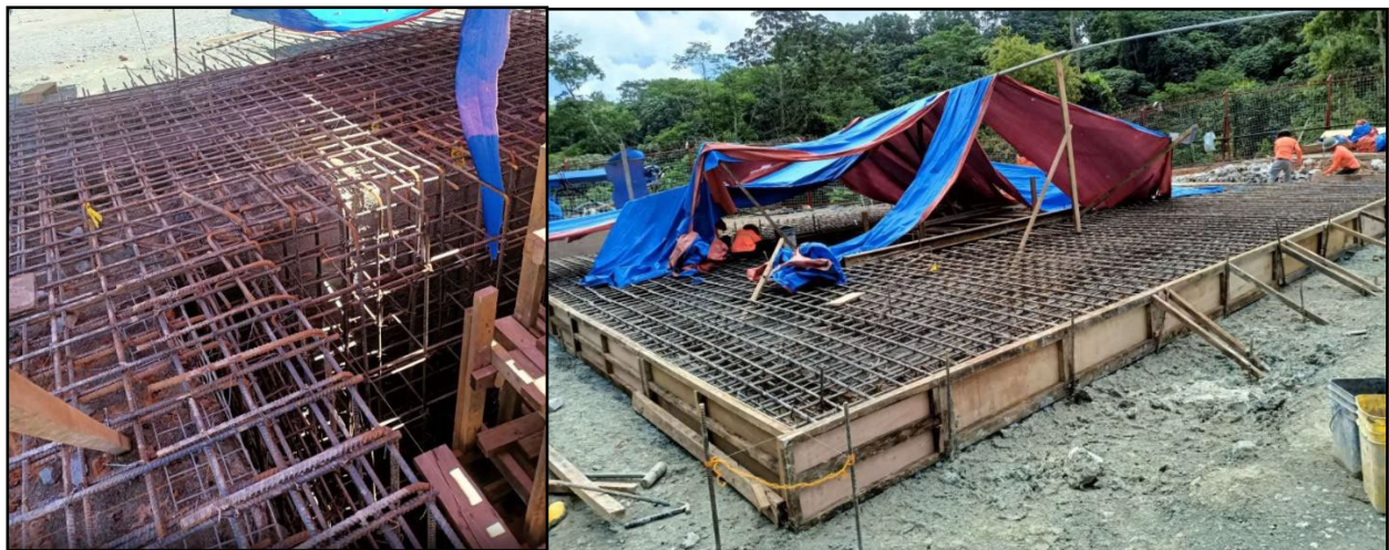
Photo 1: installation of the rebar matting and frameworks as part of the Ventilation Shaft collar preparation
