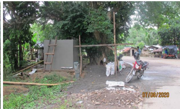
Picture 5. Water Tank Collector for water system of Nueva Era Elem. School - Nueva Era, Bunawan, BADS
