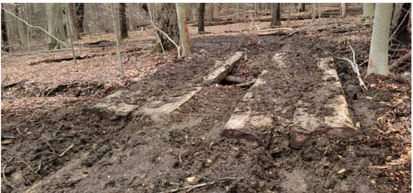
Timber mats that are not installed correctly
