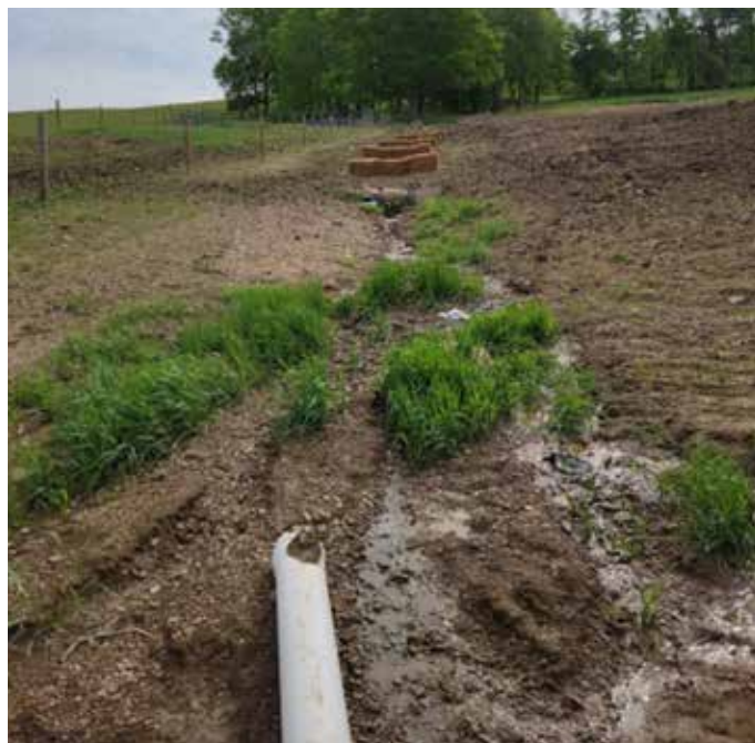
This operator is experiencing major runoff issues that are creating a gully (pictured above), eroding soil and allowing sediment to reach a nearby stream. As a temporary measure, the farmer has placed hay bales to try and slow the speed of water. ICCD is working with the farmer to create a permanent solution that will allow him to utilize the pasture.
