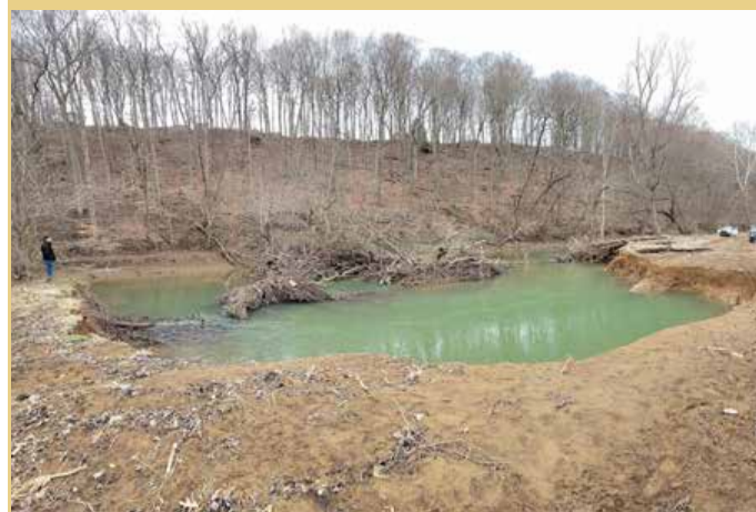
Pictured above is a crop field next to Crooked Creek that is being washed away by an eroding streambank. ICCD staff visited the site with NRCS representatives to evaluate potential solutions. Fixing this issue will require miles of streambank stabilization.
