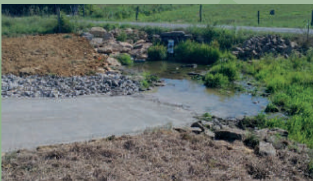
Agricultural crossing/ramp using a GP-6 permit. Stone and seeding were used for streambank stabilization.
