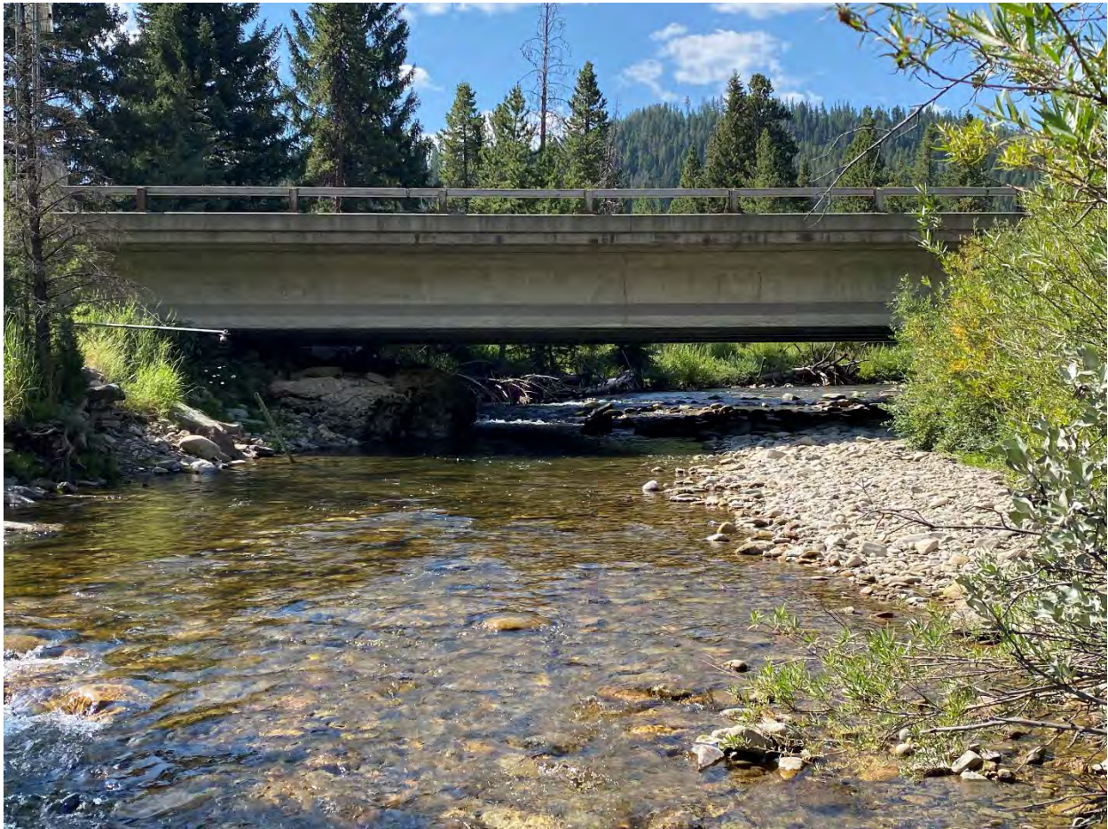
Figure 31 Bridge over the West Fork of the Gallatin River along MT-64 (Lone Mountain Trail) RM 0.2
