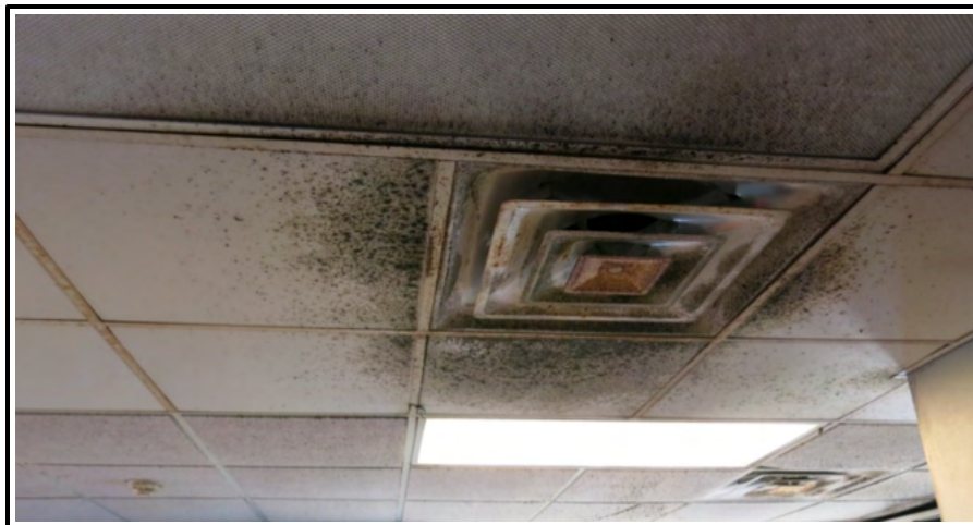
Figure 19. Mold growing near duct vents in Bldg. 2261.
