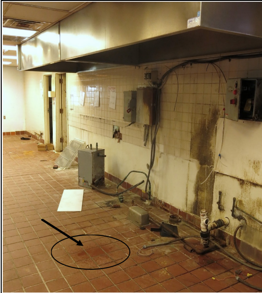
Figure 28. Leakage from ceiling piping or roofing.
