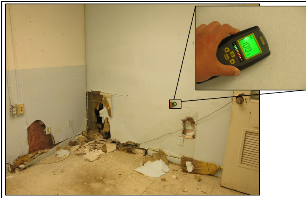
Figure 27. Wall surface moisture content of 100% near Sample Location #4.
