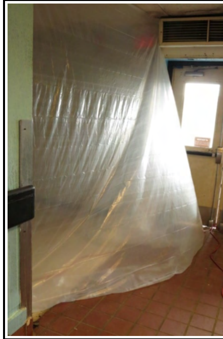
Figure 16. Positive pressure at various points within Bldg. 2261.
