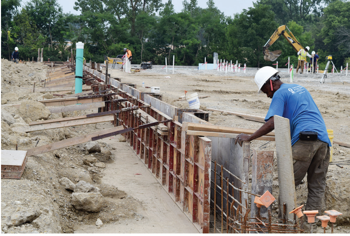
▲ Nick Price's uncle Mark Thomas, works on a concrete form at the 38th & Sheridan Project worksite.
