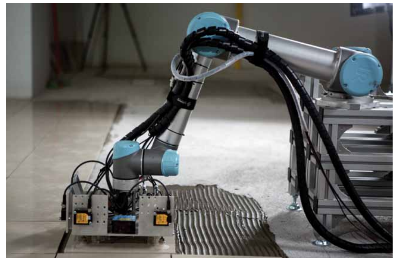
Fig. 06 Current feasibility prototype laying an area of approximately 1 m 2 . The mobile unit was moved manually around 48 times to tile an area of 30 m 2 with 300 mm x 300 mm tiles, with the robot control system re-localizing itself automatically
