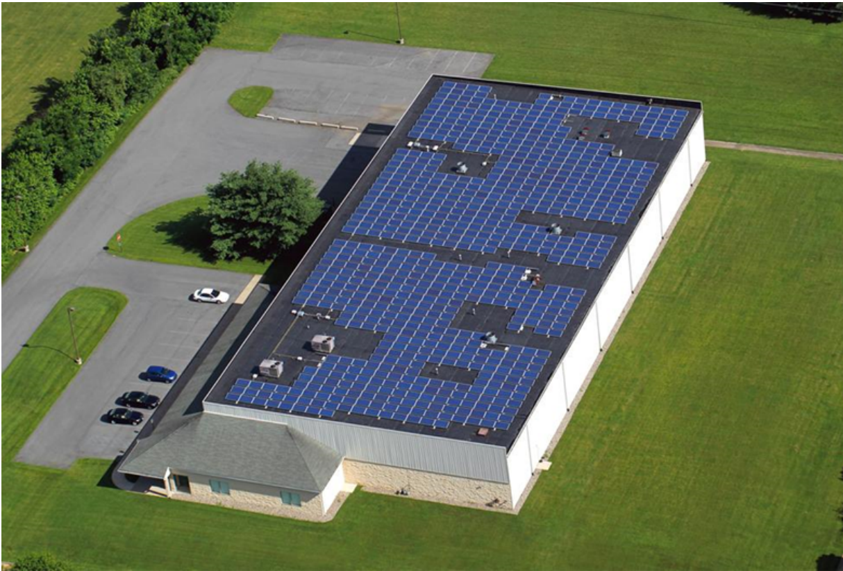
Figure 3: Commercial/industrial PV installation
