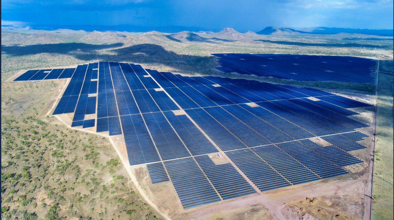
Figure 4: solar farm installation
