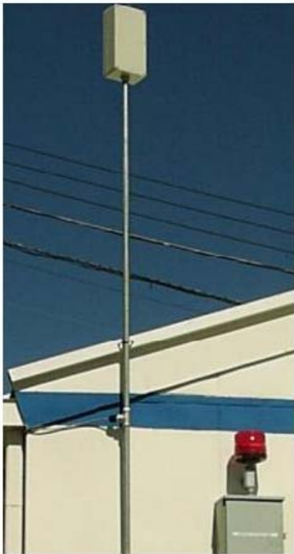
Example of receiver mount on building
