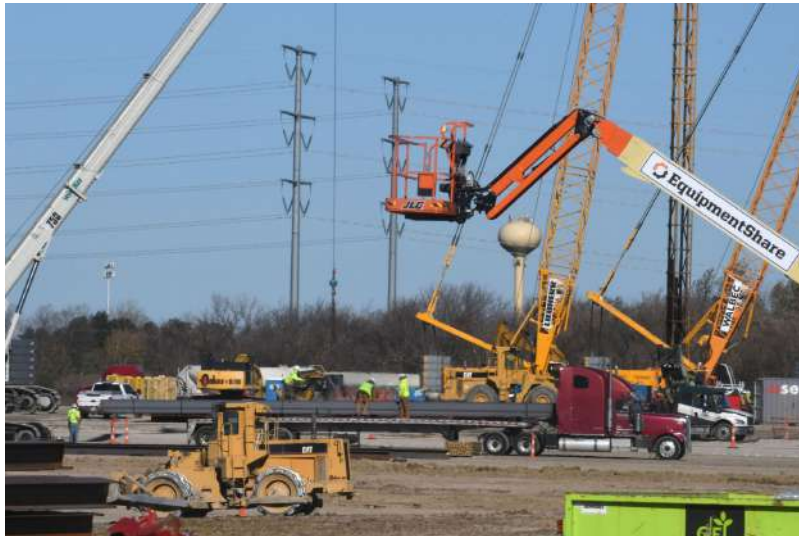
The site of a new Microsoft data center in Mount Pleasant, Wis. PHOTO: MARK HERTZBERG/ZUMA PRESS
