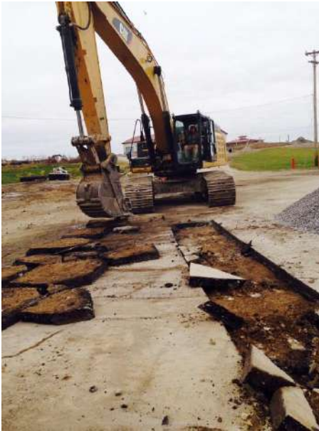
Fig.3 – Cutting pavement for the installation of sewer lines from the new maintenance building on November 11, 2015.
