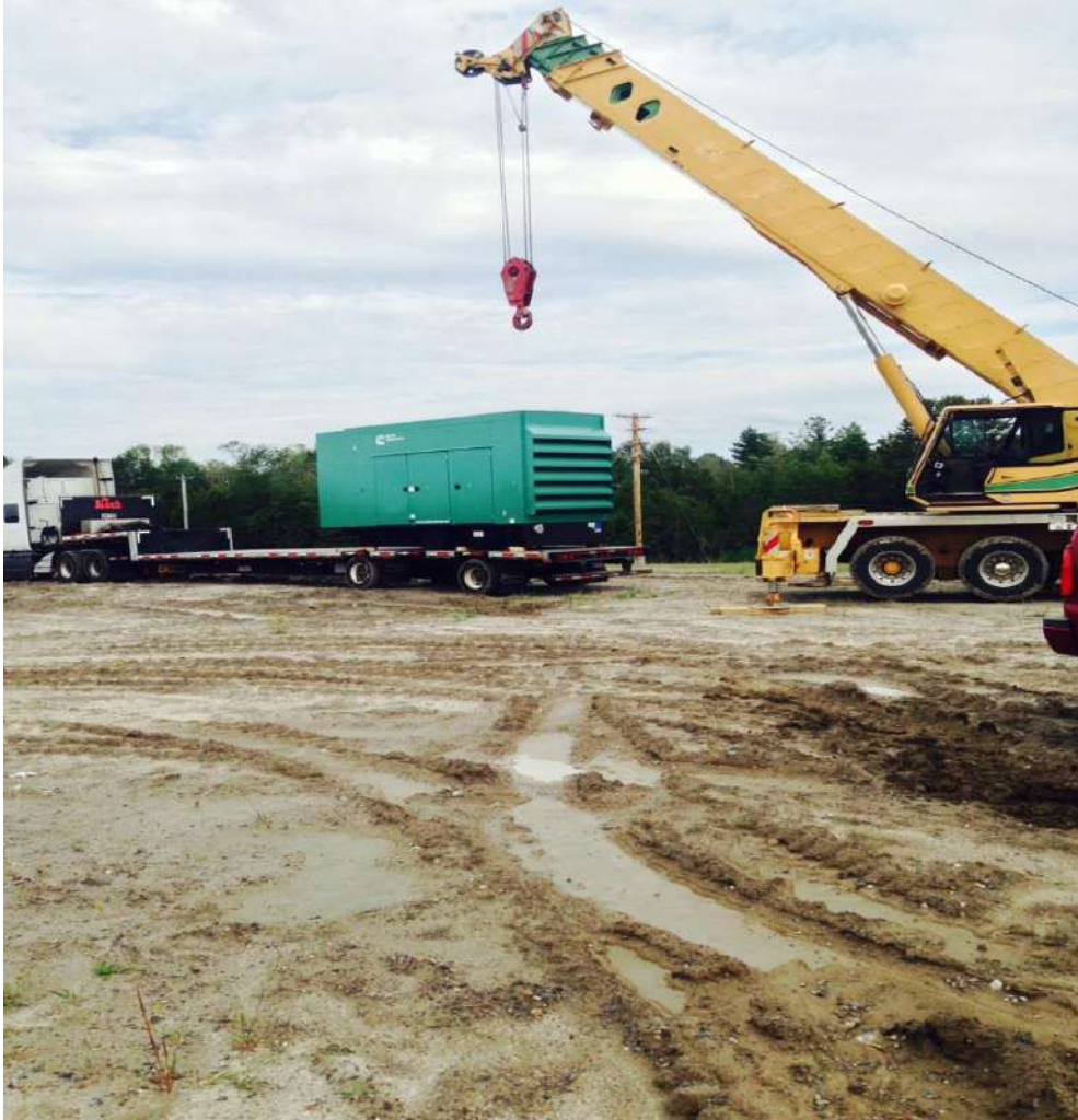
Fig. 2. Generator delivered to the Landfill on September 10, 2015.
