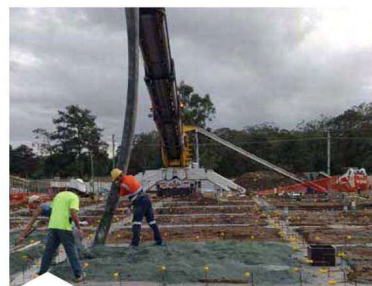
A number of chutes are available to control dust at the discharge point
