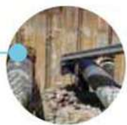
As well as bulk materials, sandbags can be handled for speedy construction of flood protection walls or creating formwork for concreting around underground infrastructure.
