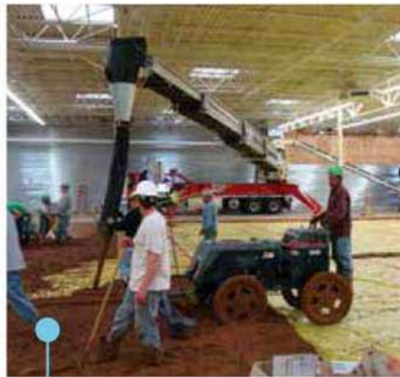
Placing concrete indoors for high productivity laser screeding equipment. A Telebelt is faster than a pump, handles stiff mixes and can work with lower head height.
