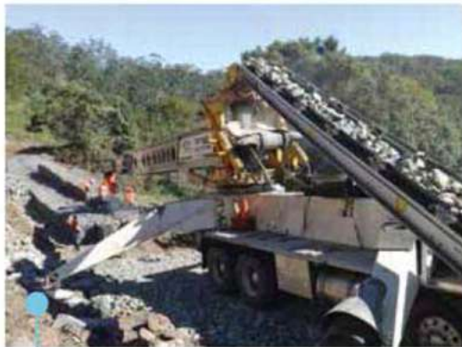
Placing stone in gabions with minimal labour requirements. Stone can be stockpiled close to road access and fed into the Telebelt hopper by excavator or loader.
