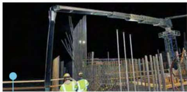
Tower-mounted Telebelt systems are an option for long-term projects or where set-up space is limited.
