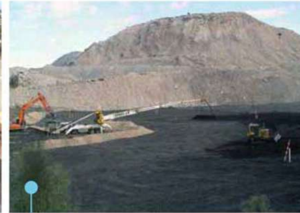
Capping a tailings dam by placing coal rejects over geotextile for a swamp dozer to push out.
