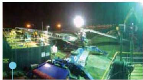
Discharging roadbase from a barge direct into articulated dump trucks for an island project. Congestion and double handling is avoided.
