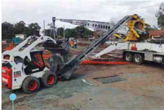
Crusher dust being loaded into a hopper for placement under a slab. A variety of hoppers is available to suit the material and loading method.
