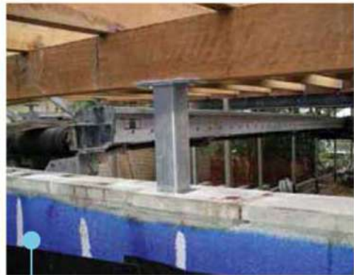
Telebelt working with restricted access to backfill behind a retaining wall. The ability to telescope and slew allows it to work around posts and other obstructions.
