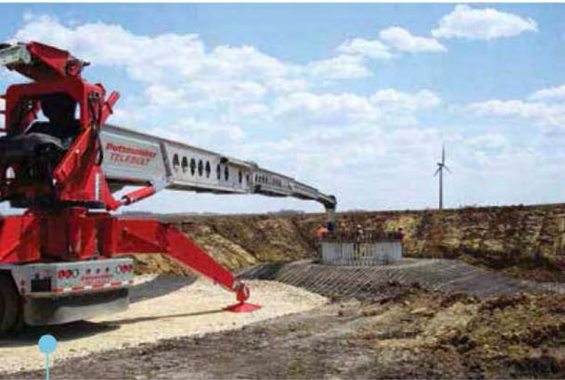
Telebelts can place concrete for the tower bases and roadbase material for site access roads at wind farm projects.
