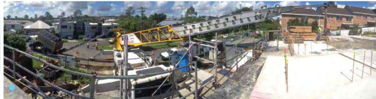
Panorama image of tipper on the street discharging directly into the feed belt hopper via a grain chute, with the telescopic placement belt used to place 20mm drainage gravel around a unit block slab at an elevated level.
