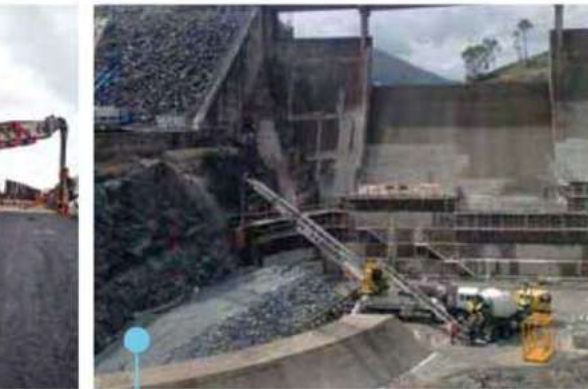
Placing concrete at a dam upgrade project. The ability to handle multiple materials and stiff concrete mixes is an asset on a remote site, compared to a pump.
