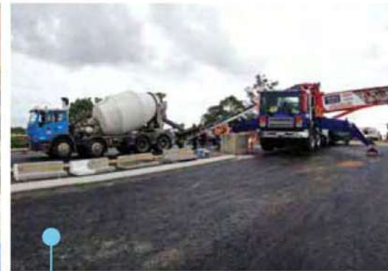
Pouring cast in situ barriers for a railway overpass. The reach of the Telebelt can generally avoid having trucks on the bridge, and minimises disruption to other works.
