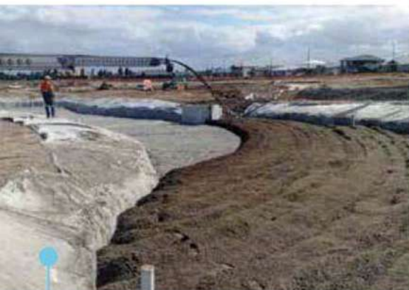
This Telebelt remained on site to place both materials over geotextile for this detention basin.
