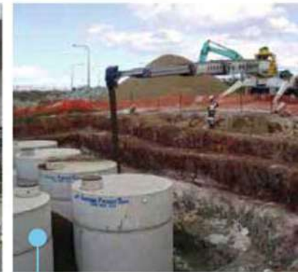
Placing backfill material around underground water tanks, where conventional earthmoving equipment cannot gain access.
