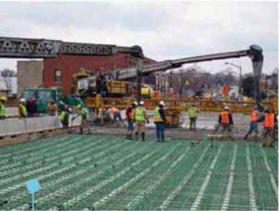
Placing concrete for bridge slabs, concrete hard stands and other large slabs. Material can be placed evenly across the slab ahead of the paver.
