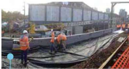
Placing no fines concrete behind precast wall panels for a rail project. Feed from two agitators speeds the placement.
