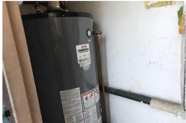
#28 GAS WATER HEATER
