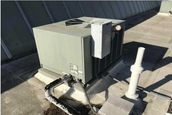
#25 SPLIT SYSTEM CONDENSING UNIT
