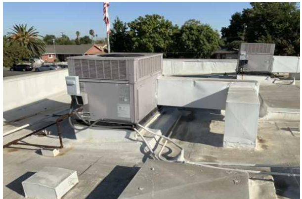
#24 PACKAGE UNIT AT ADMIN
