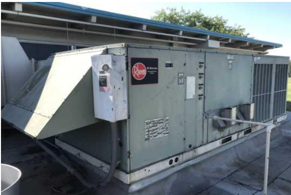
#23 PACKAGED UNIT AT MPR
