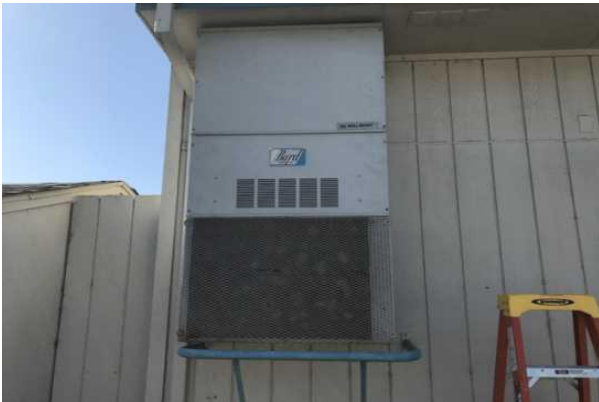
#27 HEAT PUMP AT PORTABLES
