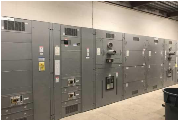
#29 MAIN ELETRICAL EQUIPMENT
