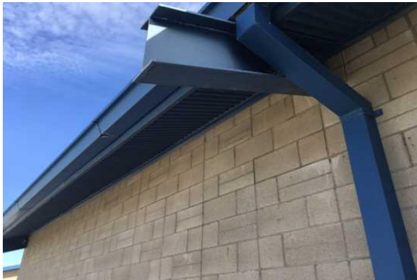
#15 LEAKY GUTTER IN BUILDING F/G ROOF
