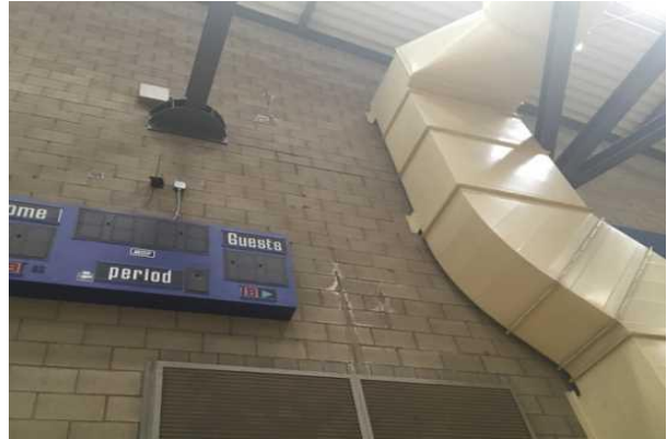
#14 MOISTURE ISSUES - INTERIOR WALL - LARGE GYM
