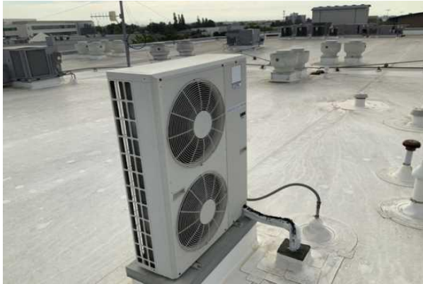
#25 DUCTLESS MINI-SPLIT UNITS
