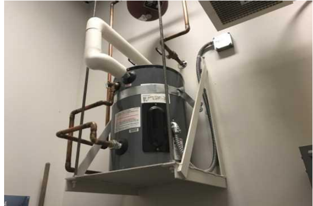
#32 WATER HEATER, ELECTRIC
