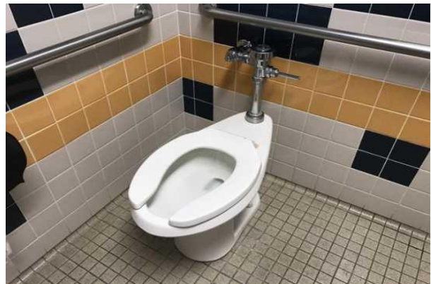
#34 TOILET, COMMERCIAL WATER CLOSET
