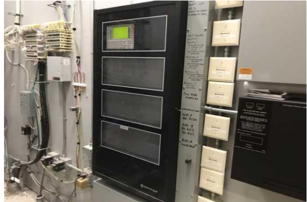
#20 FIRE ALARM PANEL
