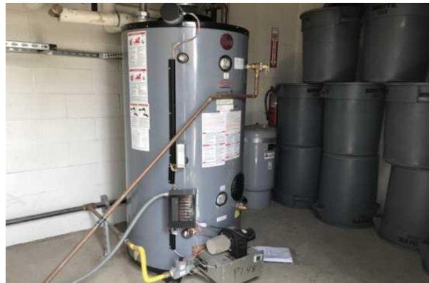
#30 DOMESTIC WATER HEATER/BOILER/STORAGE TANK
