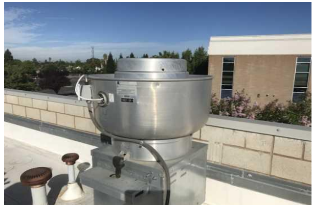
#24 TYPICAL EXHAUST FAN, ROOF
