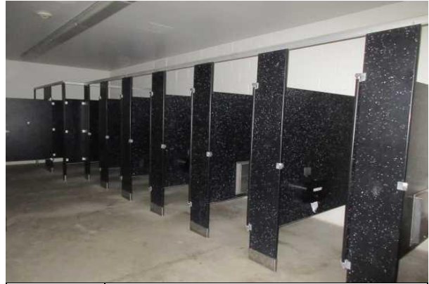
#44 TOILET PARTITIONS, METAL
