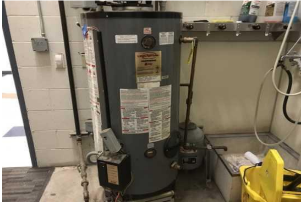
#31 WATER HEATER, GAS
