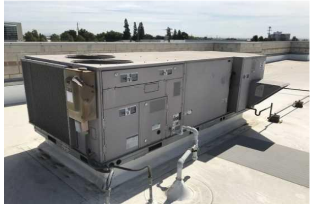
#26 PACKAGED UNIT (RTU) WITH HEAT RECOVERY
