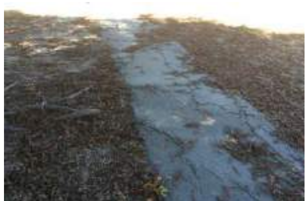
#48 CRACKED PAVEMENT NEAR PLAY STRUCTURE
