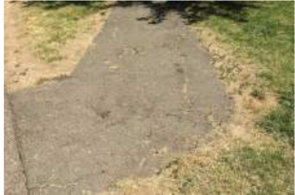
#44 ASPHALT PATH WITH CRACKS NEAR MAIN PLAYGROUND
