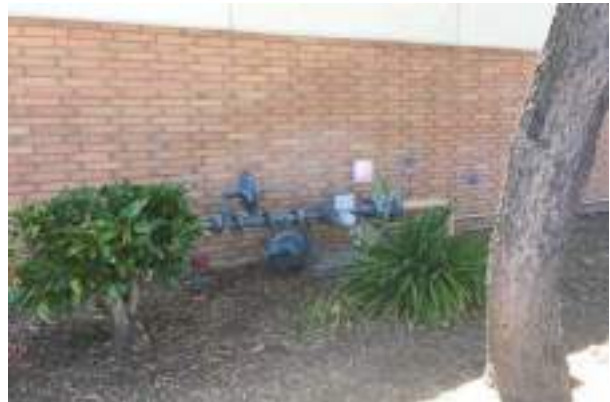
#40 NATURAL GAS METER
