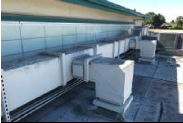
#31 HVAC SYSTEM DUCTWORK
