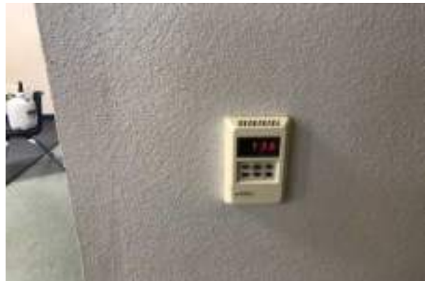
#30 LOCAL HVAC CONTROLS
