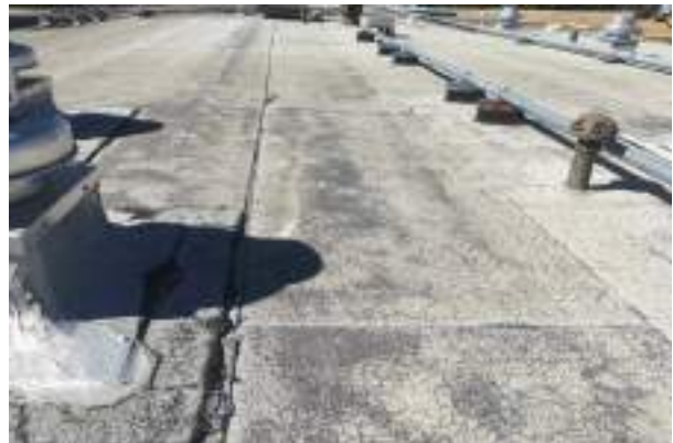
#12 MODIFIED BITUMINOUS ROOF WITH BLISTERS AND CRACKS
