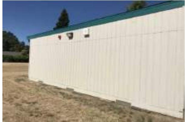
#38 FIRE ALARM EXTERIOR
