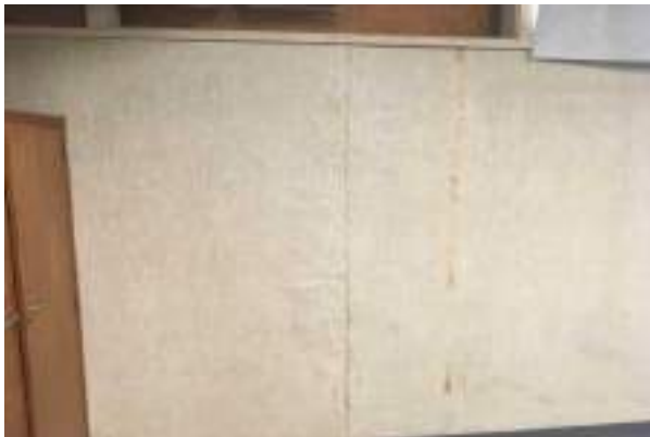
#17 WALL PAPER DAMAGED
