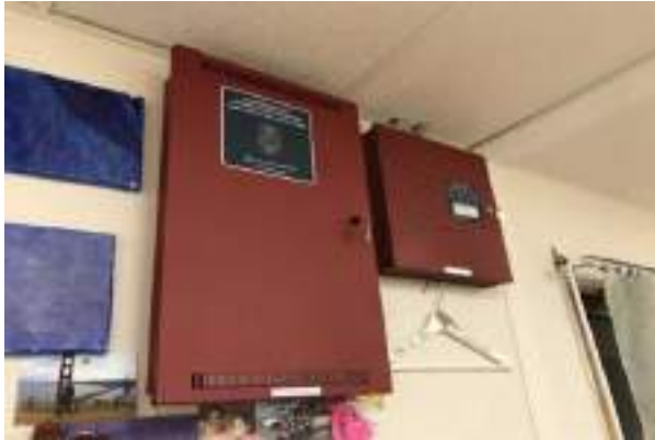
#37 MAIN FIRE ALARM PANEL
