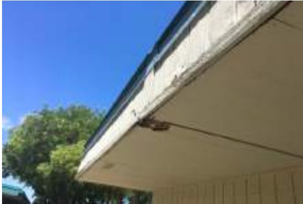
#13 DAMAGED FASCIA BOARD AND SOFFIT ON 4R PORTABLE
