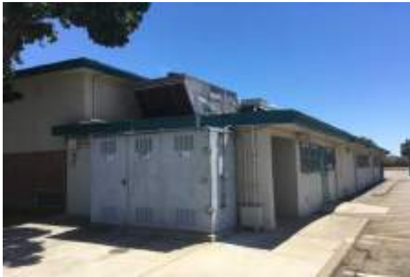
#33 MAIN ELECTRICAL SERVICE
