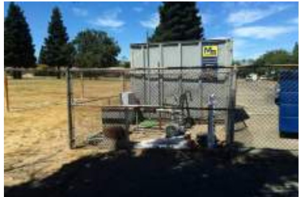
#46 IRRIGATION PUMP AND CONTROLLER
