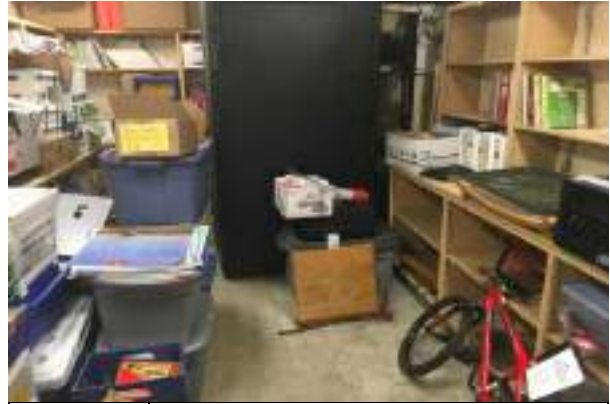
#32 STORAGE ROOM; SERVER ADDED BUT NO HVAC OR VENTING
