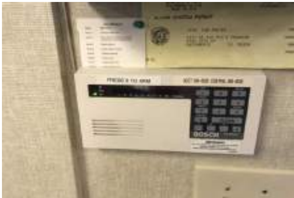
#35 SECURITY ALARM CONTROLLER (PRINCIPAL'S OFFICE)
