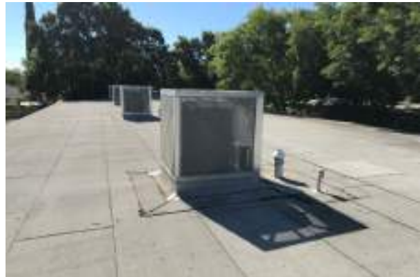
#28 CONDENSING UNITS AT ROOF
