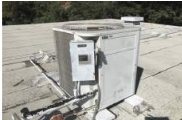
#24 CONDENSING UNIT/HEAT PUMP
