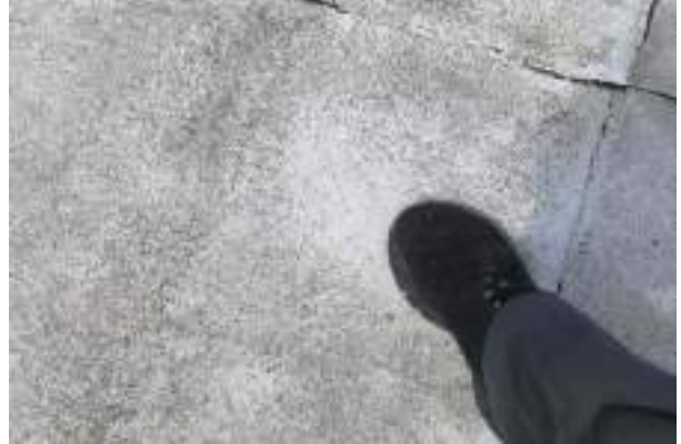
#14 BUBBLE IN ROOFING, BUILDING P02
