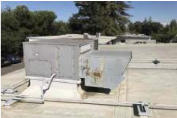
#23 ROOFTOP PACKAGED UNIT
