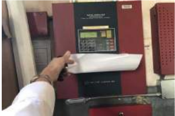
#32 FIRE ALARM CONTROL PANEL
