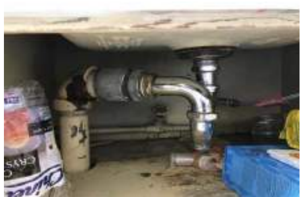
#22 ORIGINAL PLUMBING, BUILDING 2
