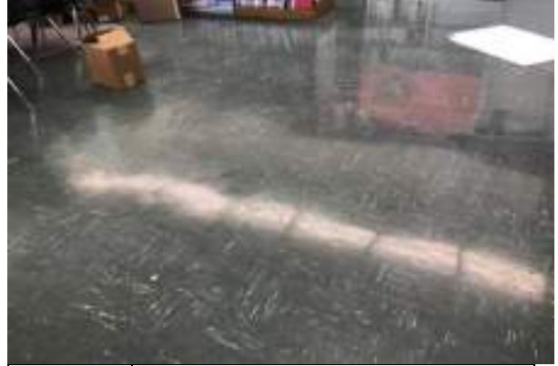
#38 VINYL-ASBESTOS FLOOR TILE IN CLASSROOM, BUILDING 1
