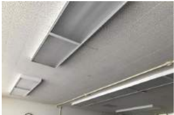
#30 LIGHTING SYSTEM, INTERIOR
