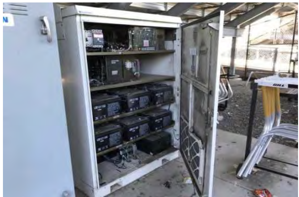
#60 UNINTERRUPTIBLE POWER SUPPLY
