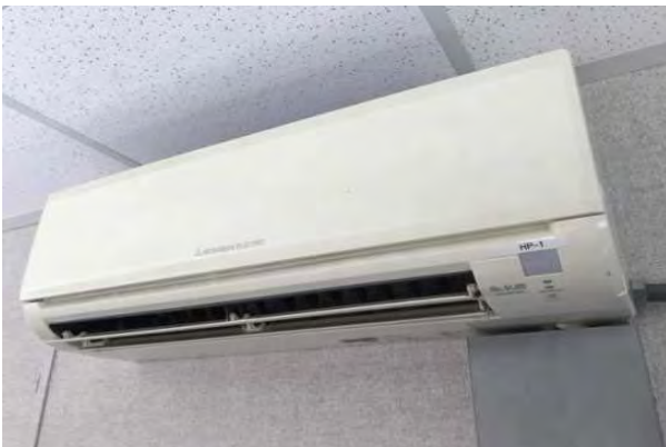
#53 DUCTLESS SPLIT SYSTEM
