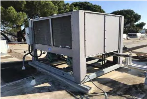
#55 AIR-COOLED CONDENSING UNIT
