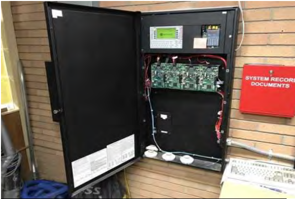
#61 FIRE ALARM CONTROL PANEL
