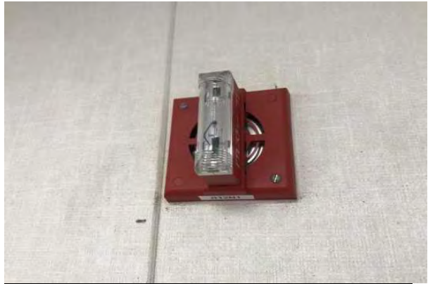
#62 FIRE ALARM SYSTEM
