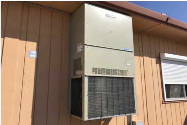
#47 WALL-MOUNTED PACKAGE UNIT
