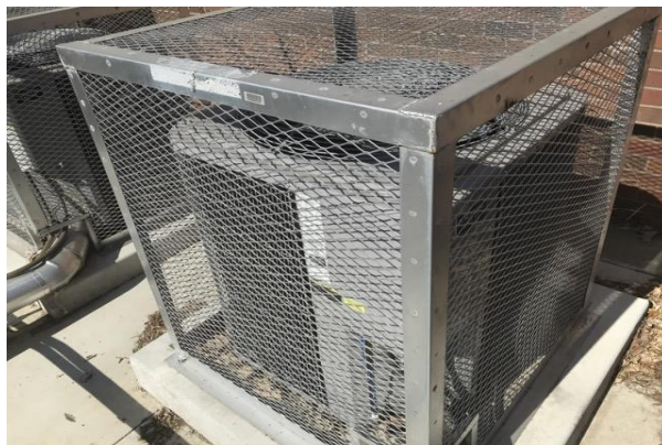
#29 CONDENSING UNIT/HEAT PUMP, SPLIT SYSTEM
