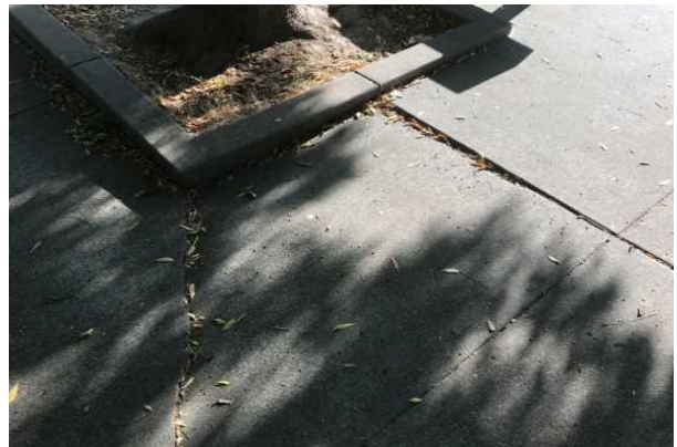
#42 TRIP HAZARDS, CENTRAL QUAD
