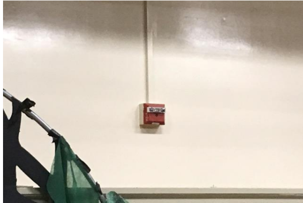
#25 FIRE ALARM SYSTEM
