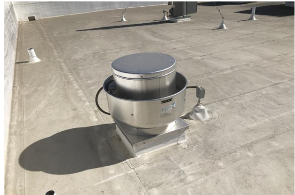
#34 EXHAUST FAN, ROOF MOUNTED
