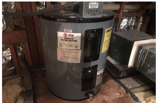
#18 WATER HEATER, ELECTRIC
