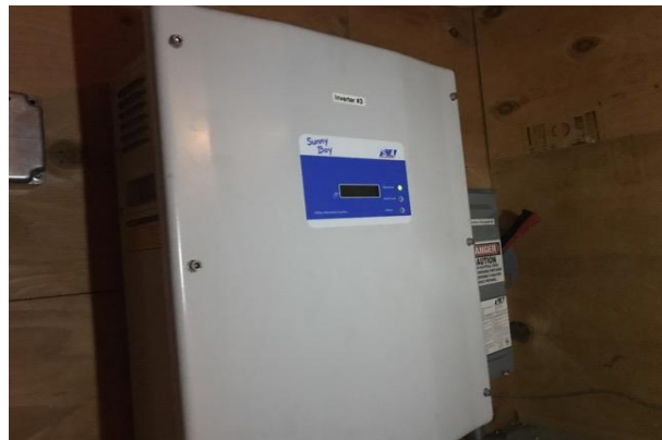
#22 SOLAR INVERTER, 7500 WATTS, REPLACE
