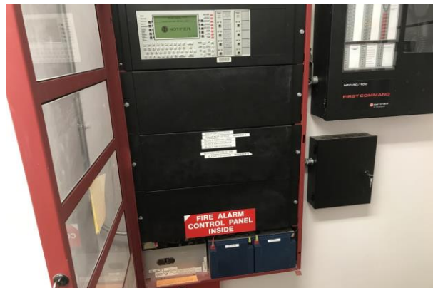
#24 FIRE ALARM CONTROL PANEL
