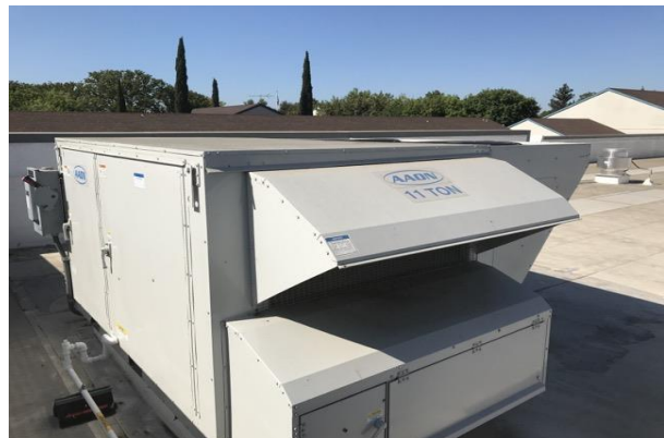
#28 PACKAGED UNIT (RTU)
