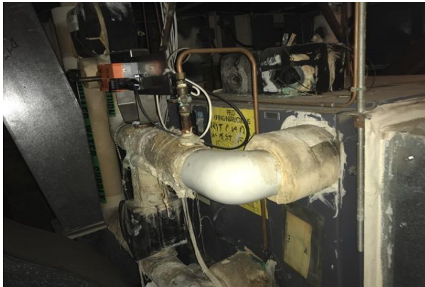
#33 AIR HANDLER (AHU), INTERIOR
