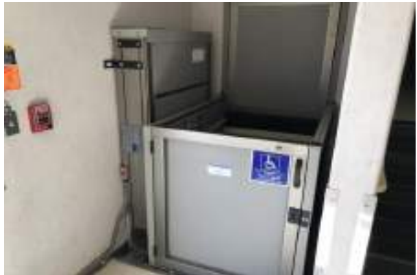
#40 WHEELCHAIR LIFT MPR BUILDING
