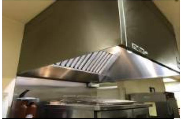
#56 KITCHEN EXHAUST HOOD
