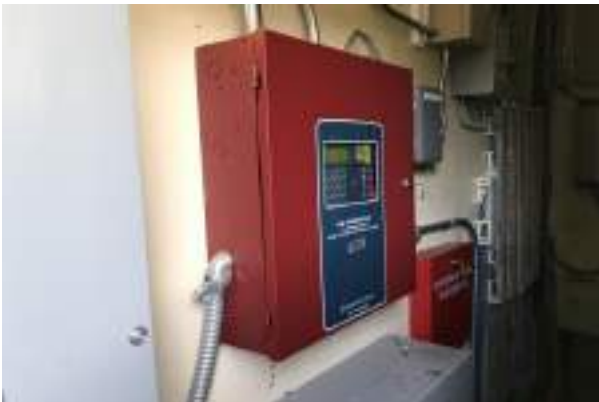
#41 FIRE ALARM CONTROL PANEL
