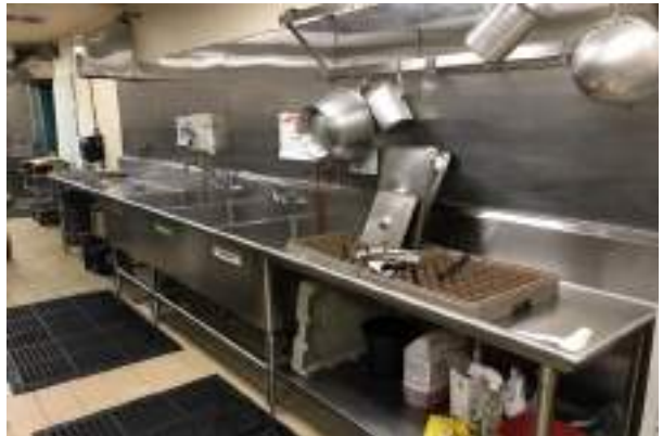
#52 KITCHEN STAINLESS STEEL SINK
