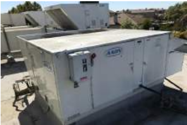
#29 PACKAGED UNIT (RTU) MPR
