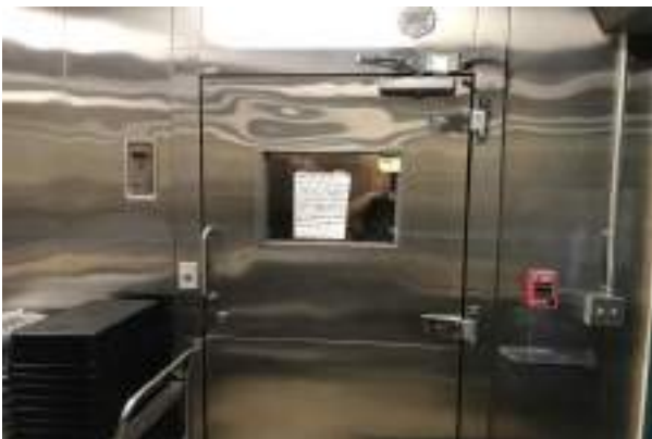
#53 KITCHEN WALK-IN FREEZER
