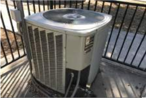
#31 CONDENSING UNIT/HEAT PUMP, SPLIT SYSTEM
