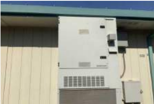
#27 PACKAGED HEAT PUMPS- PORTABLES
