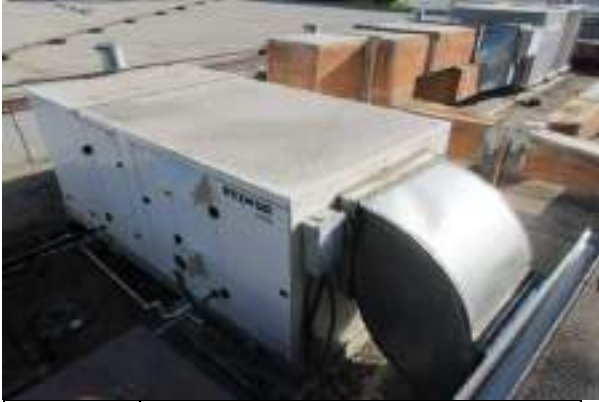
#25 AIR HANDLER- B001
