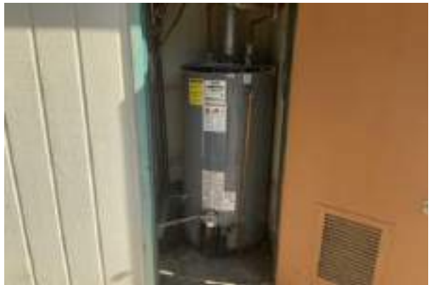
#30 WATER HEATER B-001
