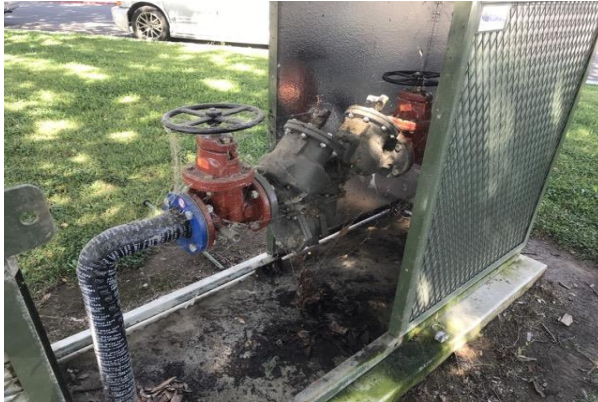
#19 BACKFLOW PREVENTER, DOMESTIC
