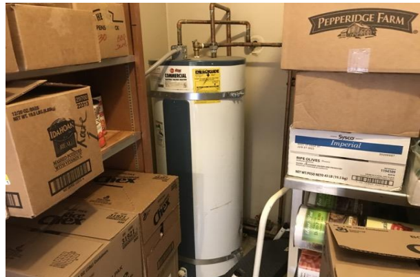
#18 WATER HEATER, ELECTRIC, COMMERCIAL
