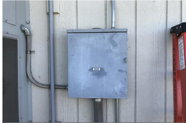
#26 MAIN DISTRIBUTION PANEL
