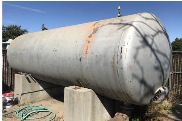
#30 AGING IRRIGATION WATER STORAGE TANK
