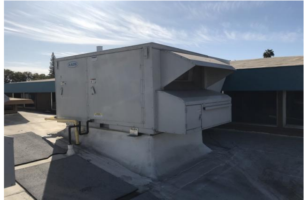
#20 PACKAGED UNIT (RTU)
