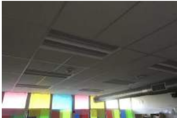
#33 C WING AND D WING, LED LIGHTING SYSTEM
