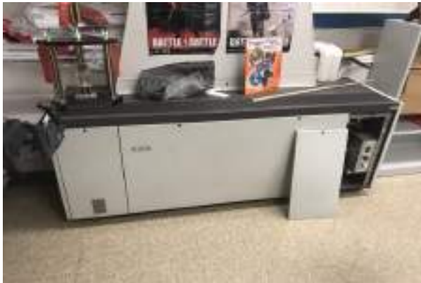
#45 001 A AND B WING, CLASSROOM UNIT VENTILATOR
