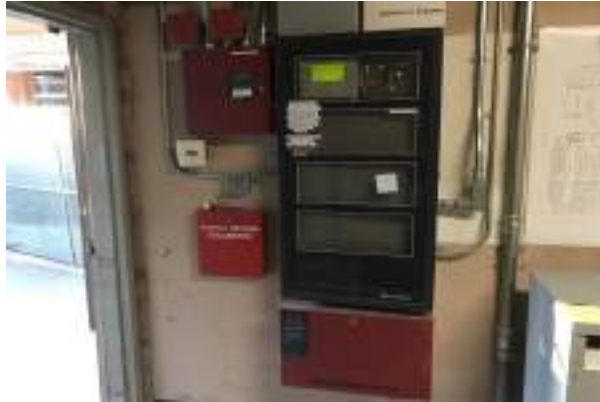
#55 001 A WING, B WING, FIRE ALARM CONTROL PANEL, BASIC/ZONED
