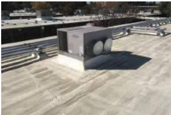
#51 HEATING AND CHILLED WATER PIPING ON ROOF
