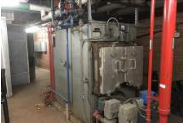
#43 16A AUDITORIUM, DOMESTIC BOILER, GAS
