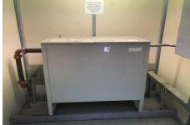
#32 P02 X04-X08, ELEVATOR, HYDRAULIC
