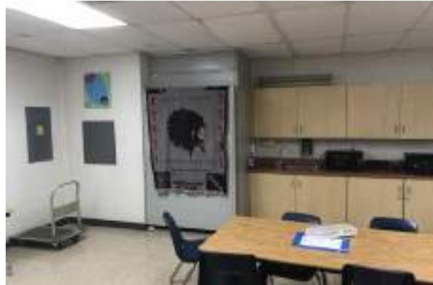
#50 P01-P03, CLASSROOM HEAT PUMP
