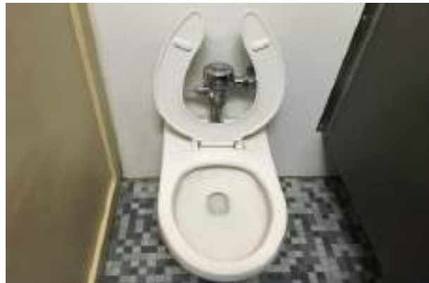
#36 TOILET, COMMERCIAL WATER CLOSET
