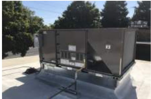
#46 C-F WING, ROOFTOP PACKAGED UNIT
