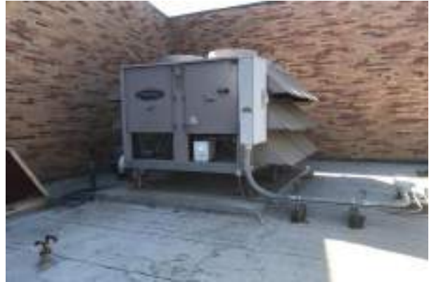
#44 16A AUDITORIUM, CHILLER, AIR-COOLED
