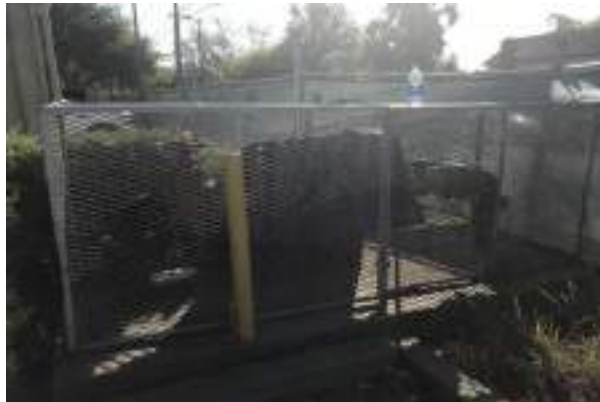
#39 BACKFLOW PREVENTER, DOMESTIC
