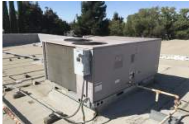
#48 015 CAFETERIA, ROOFTOP PACKAGED UNIT (RTU)
