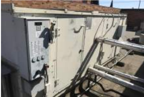
#49 16B ROOFTOP, AIR HANDLER (AHU), EXTERIOR
