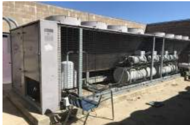
#42 013 ROTC, CHILLER, AIR-COOLED
