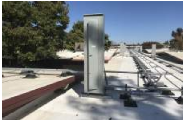
#54 C WING - F WING, ROOFTOP MAIN DISTRIBUTION PANEL
