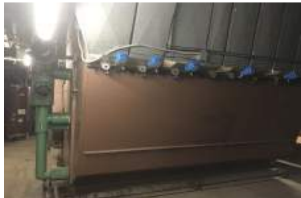
#52 16A AUDITORIUM, AIR HANDLER (AHU), INTERIOR
