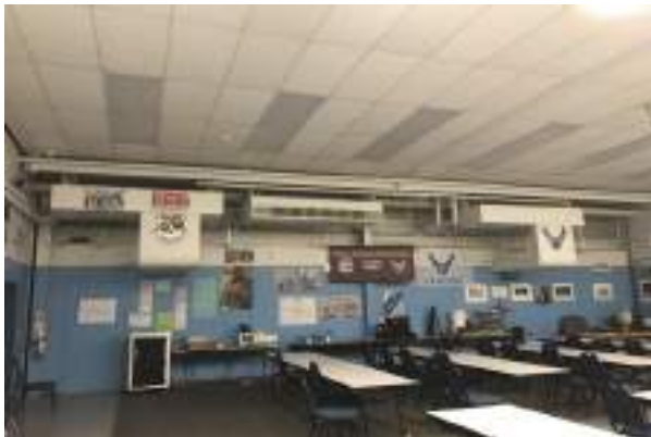
#47 011 AND 012 S WING, UNIT VENTILATOR
