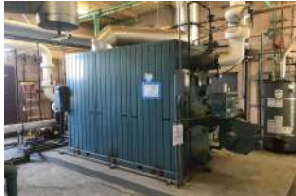
#40 013 ROTC, HEATING HOT WATER PLANT BOILER
