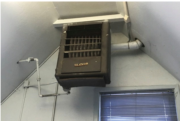
#27 UNIT HEATER, BUILDING 5
