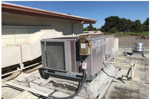
#24 PACKAGED UNIT (RTU), BUILDING 2
