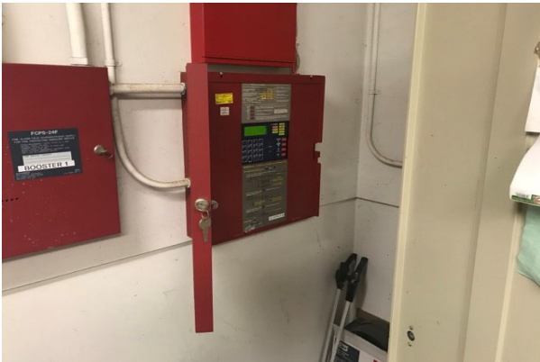
#33 FIRE ALARM CONTROL PANEL
