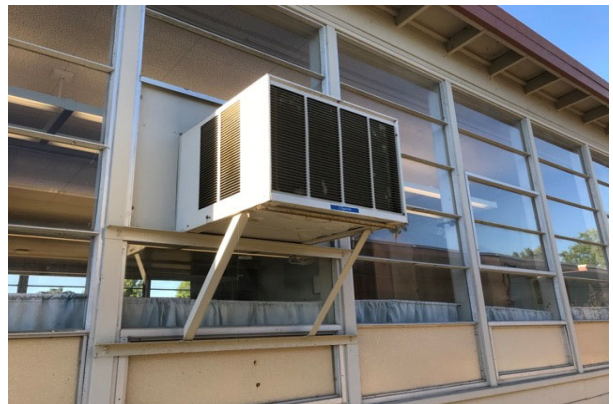
#28 AIR CONDITIONER, WINDOW/THRU-WALL, 1.5 TO 2 TON, REPLACE
