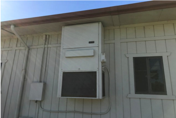
#25 HEAT PUMP, WALL-MOUNTED, BUILDING P02-3-4
