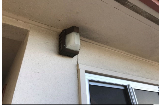
#32 EXTERIOR LIGHT FIXTURE
