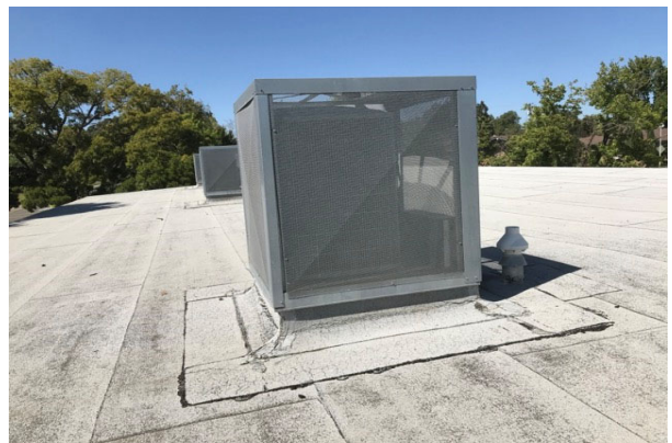
#30 ROOFTOP CONDENSING UNITS
