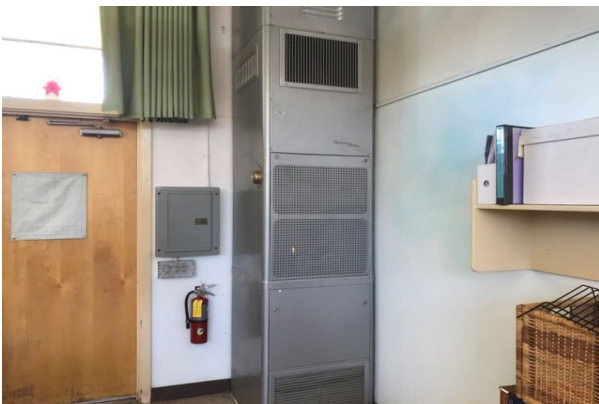
#29 FURNACE, BUILDING P01
