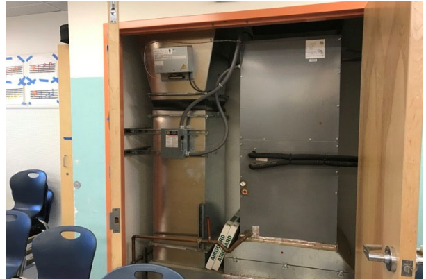
#26 FAN COIL UNIT, BUILDING P06
