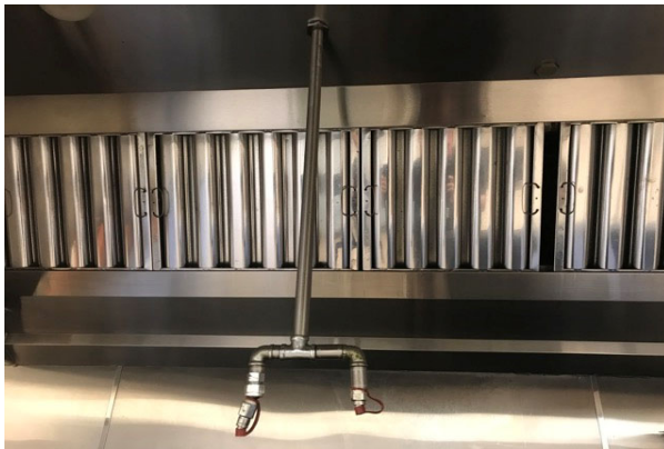
#41 D40 FIRE SUPPRESSION SYSTEM, COMMERCIAL KITCHEN
