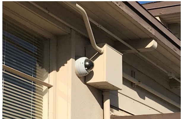
#48 D55 SECURITY/SURVEILLANCE SYSTEM, CAMERAS AND CCTV
