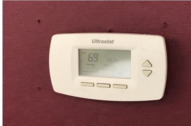
#32 D30 DEFICIENCY BAS/HVAC CONTROLS
