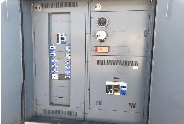
#43 D50 MAIN SWITCHBOARD
