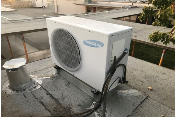
#31 D30 CONDENSING UNIT/HEAT PUMP, SPLIT SYSTEM
