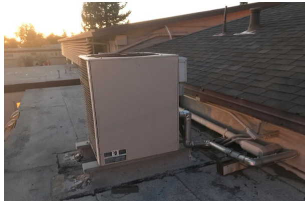
#30 D30 CONDENSING UNIT/HEAT PUMP, SPLIT SYSTEM
