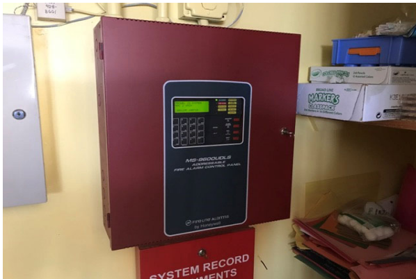
#47 D55 FIRE ALARM CONTROL PANEL
