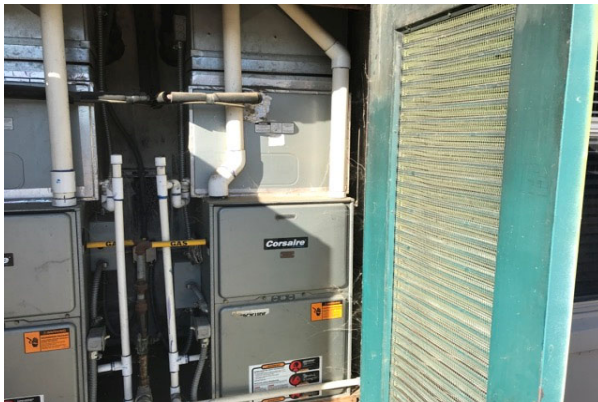
#35 D30 FURNACE, GAS
