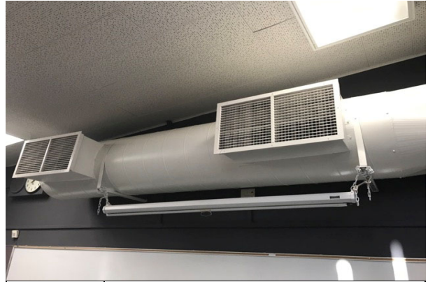
#38 D30 HVAC SYSTEM DUCTWORK
