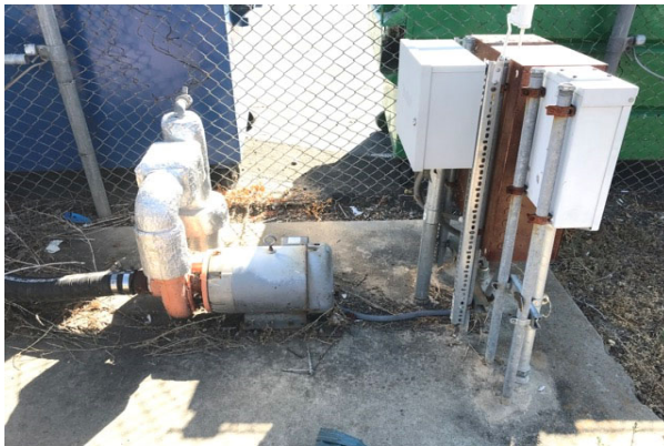
#23 D20 PUMP, DOMESTIC WATER
