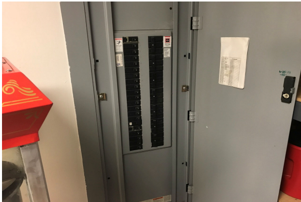
#45 D50 MAIN DISTRIBUTION PANEL
