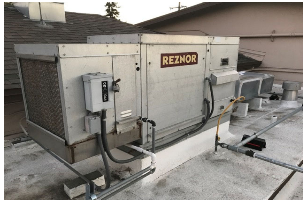
#36 D30 MAKE-UP AIR UNIT
