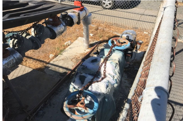
#20 D20 BACKFLOW PREVENTER, DOMESTIC
