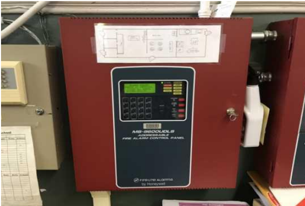
#17 FIRE ALARM CONTROL PANEL, BASIC/ZONED
