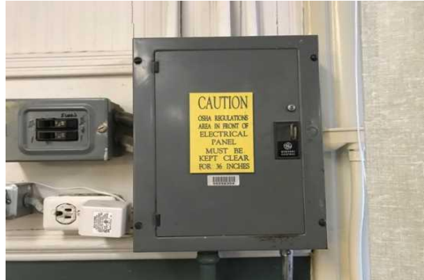
#16 MAIN DISTRIBUTION PANEL
