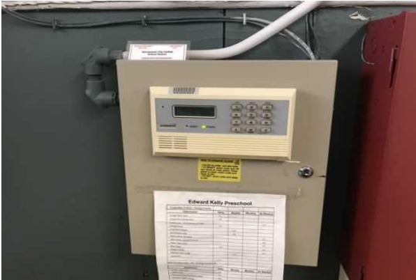
#15 INTRUSION DETECTION ALARM SYSTEM
