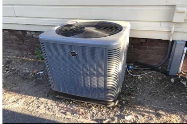
#14 CONDENSING UNIT, SPLIT SYSTEM
