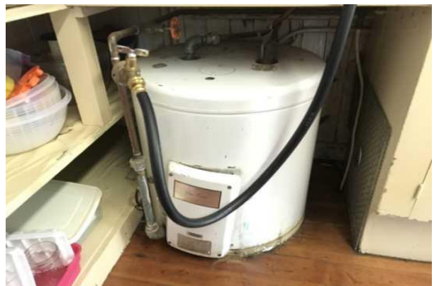
#12 WATER HEATER, ELECTRIC
