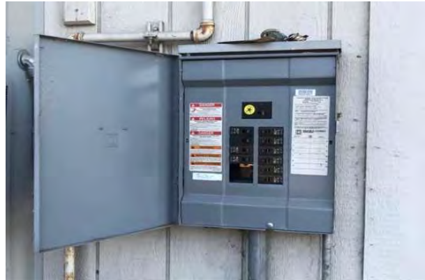
#68 PORTABLE MAIN DISTRIBUTION PANEL
