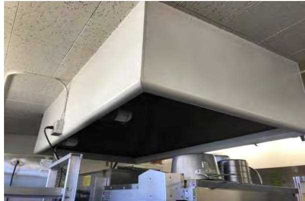
#74 KITCHEN EXHAUST HOOD
