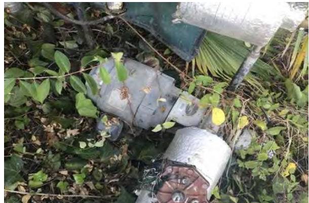
#58 DOMESTIC WATER BOOSTER PUMP
