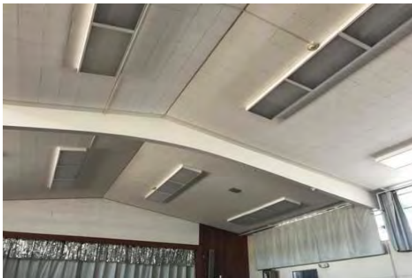
#71 T-8 LIGHTING SYSTEM
