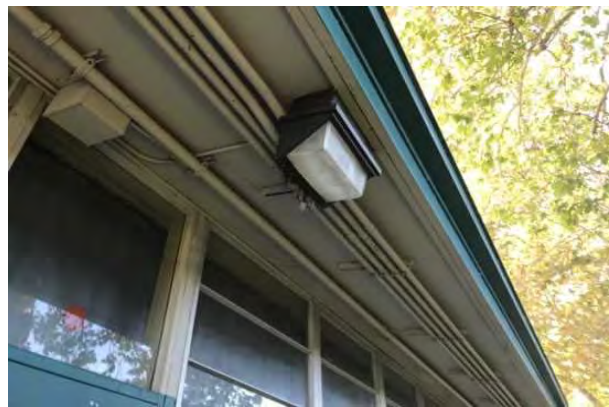
#70 EXTERIOR FLOOD LIGHT
