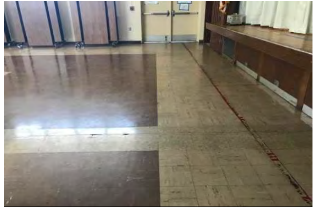
#44 MISMATCHED VINYL TILE (VCT)
