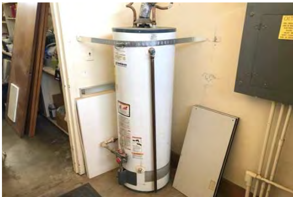
#59 GAS WATER HEATER
