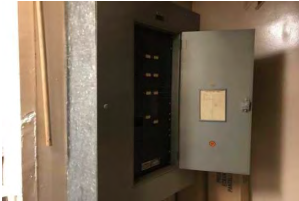
#67 001 MAIN DISTRIBUTION PANEL
