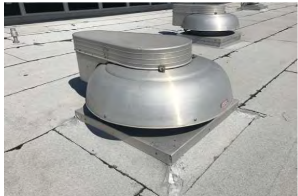
#60 KITCHEN EXHAUST FAN
