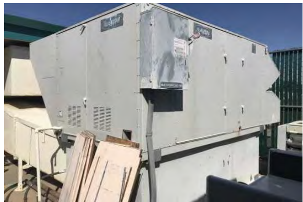
#64 MULTI-PURPOSE ROOM PACKAGED UNIT
