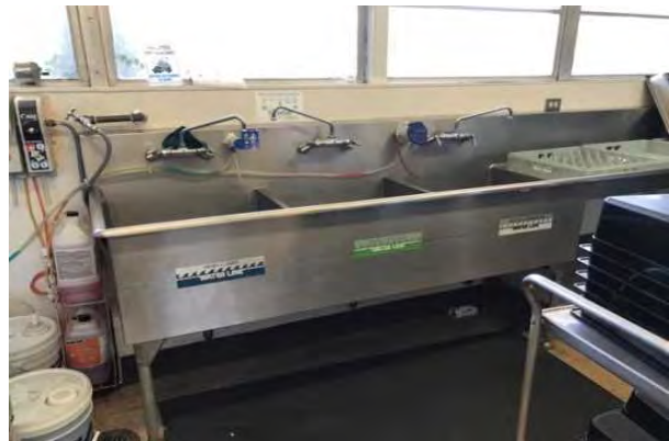
#54 COMMERCIAL KITCHEN SINK
