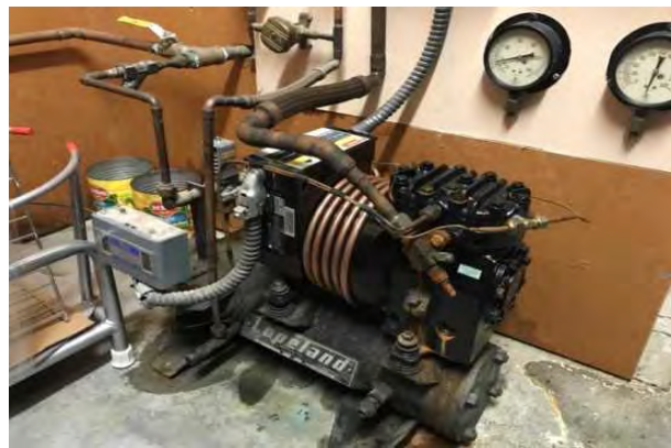
#76 WALK-IN REFRIGERATOR CONDENSER
