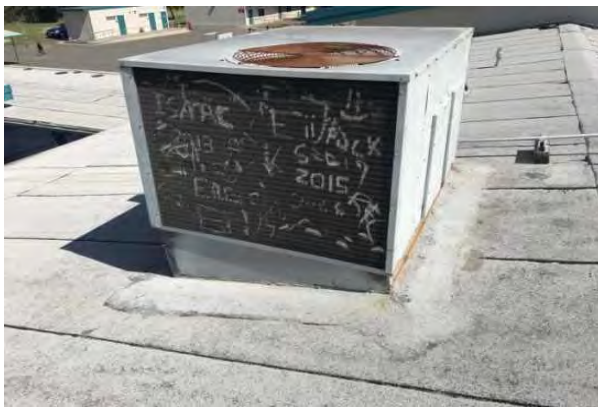
#63 PACKAGED UNIT (RTU)
