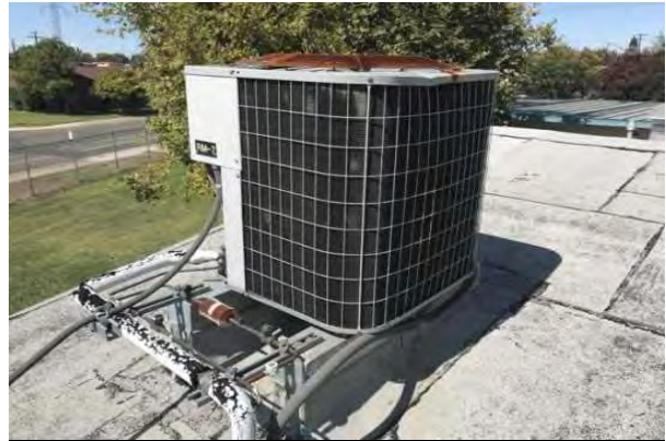
#62 SPLIT SYSTEM UNIT
