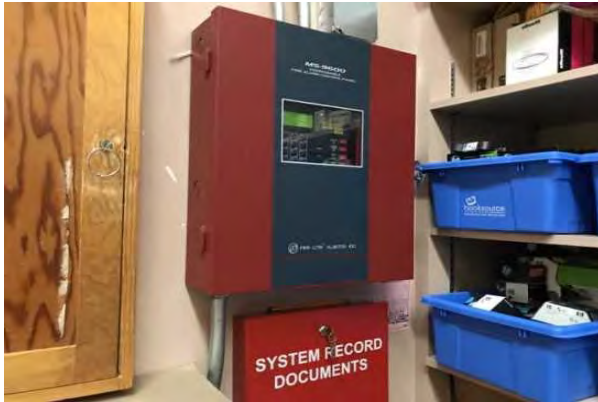
#73 FIRE ALARM CONTROL PANEL
