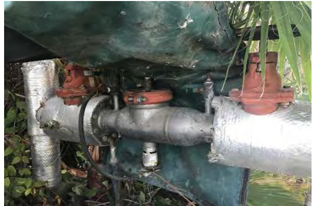
#56 DOMESTIC BACKFLOW PREVENTER
