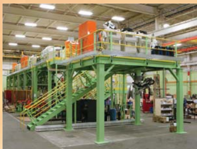
Manufacturing Mezzanine with Gantry Robot
