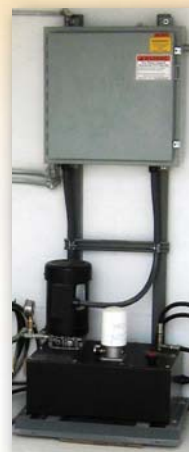
Hydraulic Pump System with control panel
