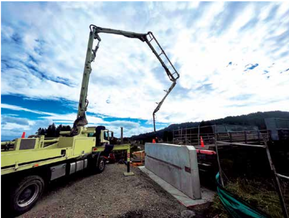
Concrete is pumped for the new abutments for the replacement rail overbridge in Ohakune.
