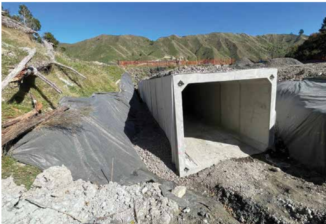
The culvert at the Auraki Stream has been extended to allow works on the road relocation.
