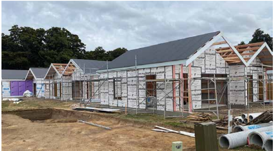
Construction of Council's six new Government COVID19 response infrastructure funded social housing units in Moore St Ohakune is proceeding well with the project on target for completion in August. It is hoped the successful delivery of this project will unlock further investment toward implementation of Council's 5-year Housing Strategy and Plan Action for addressing Ruapehu's housing issues. Photo supplied.
