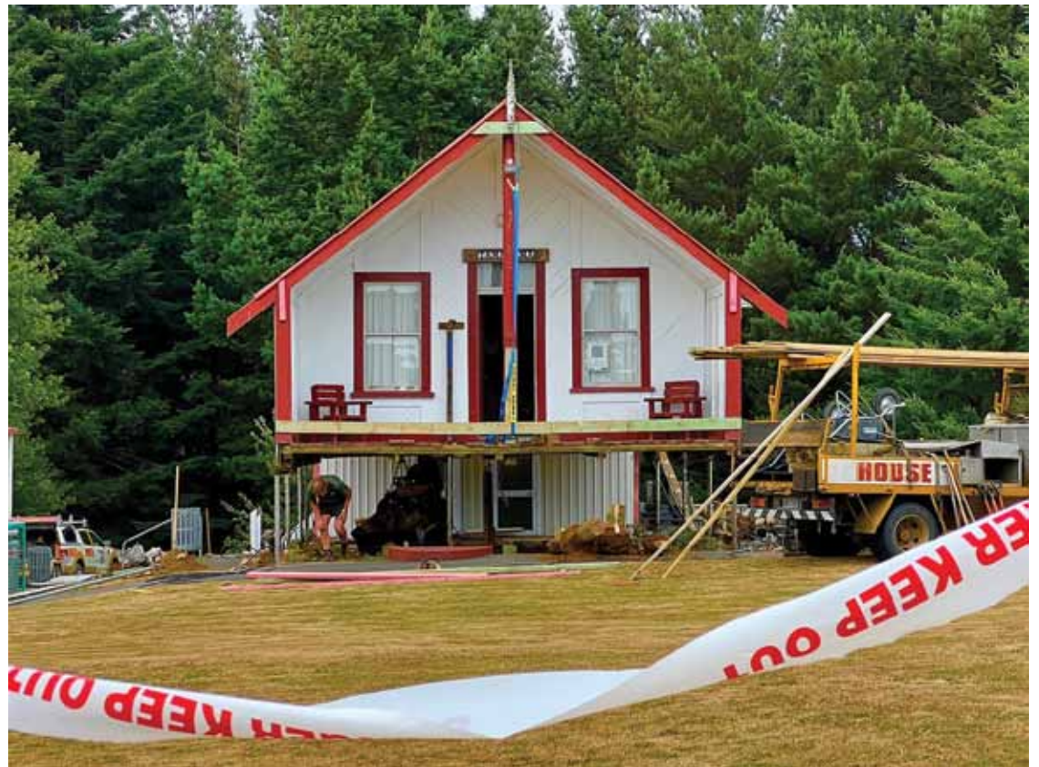
Mangamingi Marae, on the Raetihi-Ohakune Road, is lifted up to be repiled last week – part of the PGF project. Photo: Liz Brooker, Toi Communications.
