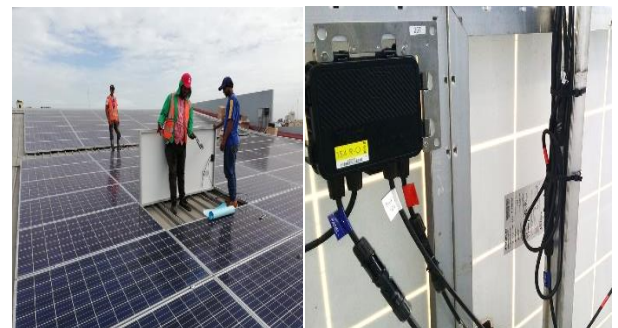
Tigo TS4-R-O units are installed on the back of each module for shade and mismatch mitigation.
