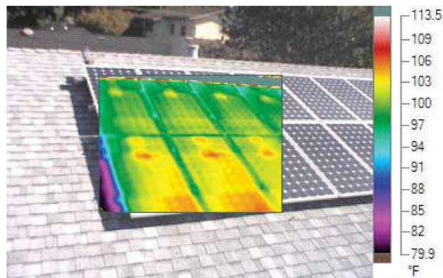
Figure 1 - Thermal image of microinverter indicating excessive heating of PV cells. It damages performance and longevity of the solar module, in addition to stressing the Microinverter components.
