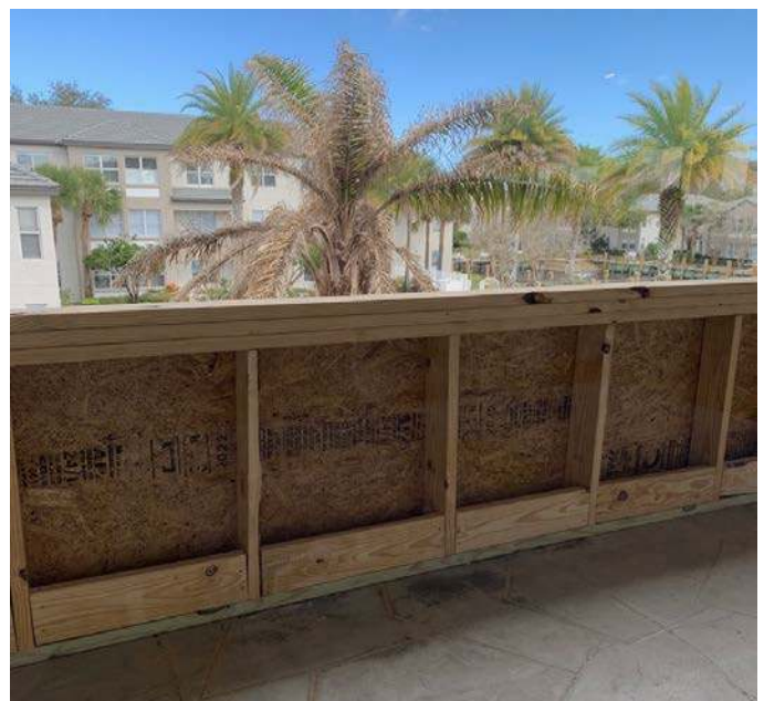
Views of the wall from outside the Coleman Center and inside LakeView.
