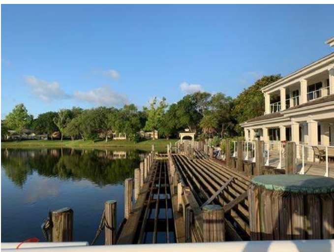
Work is well underway on these two sections further along the dock area.
