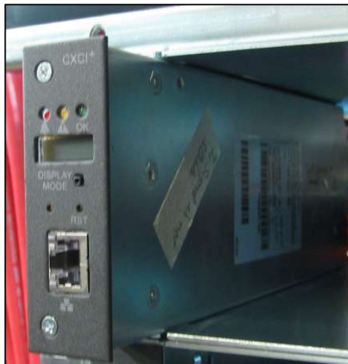
Figure 13—Cordex CXCI+ controller module
