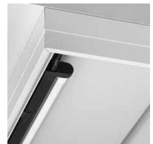
Fluorescent Light Fixture with Aluminum Light Valance
