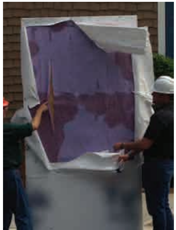
Spray rack testing shows how moisture intrusion can spread under the house wrap layer.
