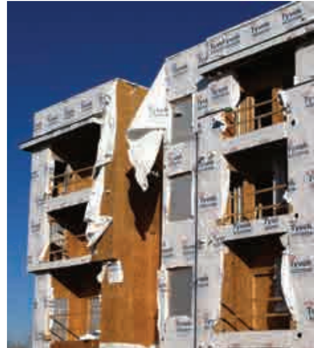
In the event that the housewrap layer is compromised all underlying sheathing could then be exposed to moisture.
